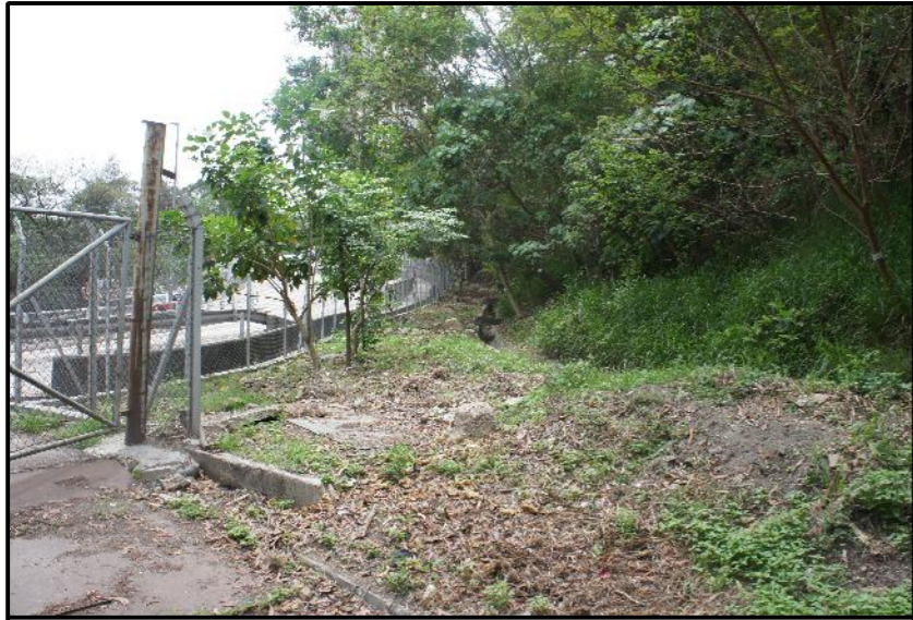
LR8.5 ENGINEERED SLOPE ALONG WITH SEMI-NATURAL DENSE HILLSIDE VEGETATION - ENGINEERED SLOPE ALONG SAU MAU PING ROAD
