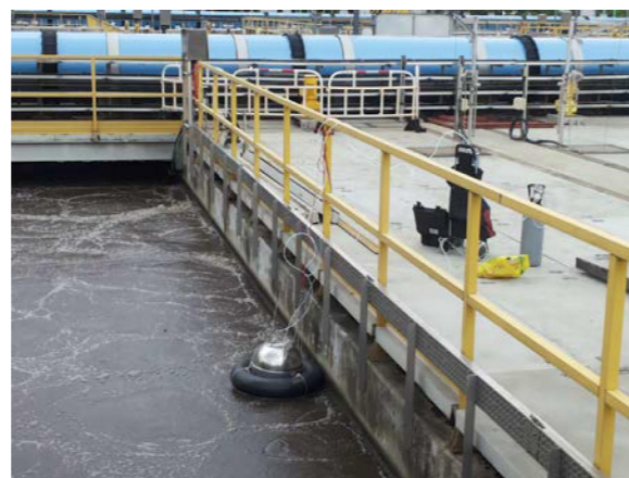
F8 - Aeration Tank (Aerobic Zone)
