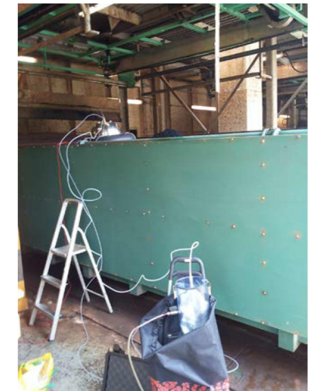
F12 - Dewatered Sludge Skip
