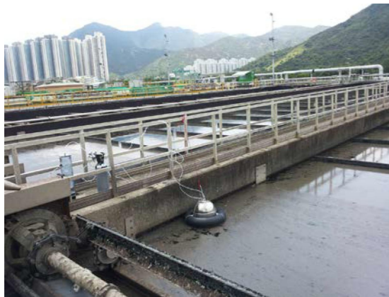
F5 - Primary Sedimentation Tank
