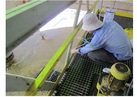
A2 - SAS Holding Tank
