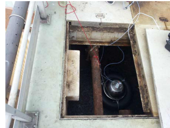
F11 - Digester Overflow Box
