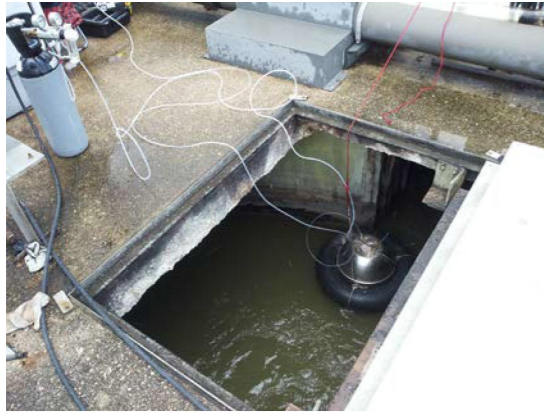
F3 - Aerated Grit Channel
