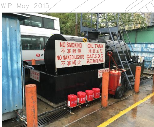
ABOVEGROUND DIESEL TANK & STEEL CONTAINMENT BUND
