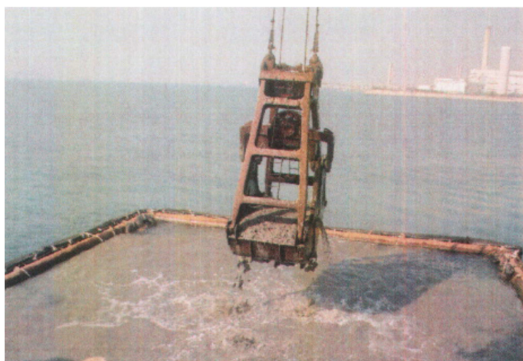
Figure 6-5: Cage Type Silt Curtain
