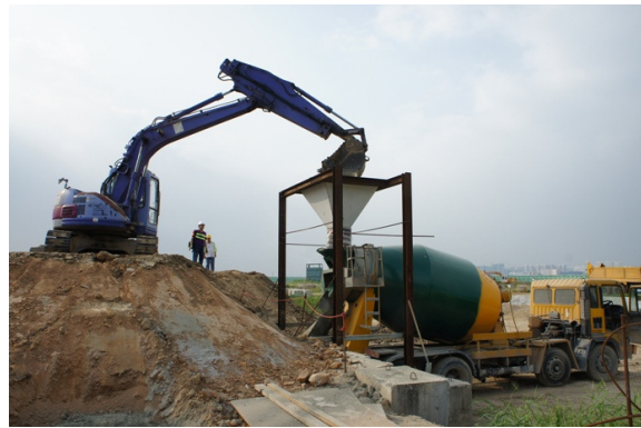
Photo 03 – Excavator and lorry mixer were utilized for handling and mixing the contaminated soil.
