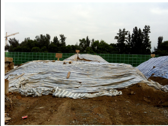
Photo 01 – The treated soil was covered with tarpaulin sheet and placed at a paved area for temporary storage.
