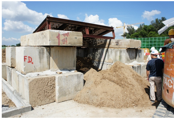
Photo 01 – The soil was screened by passing through a 35 mm sieve screening platform prior to the cement solidification process.
