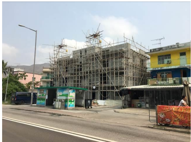
NSR P08. Village house near RCP opposite to bus stop (under construction)
