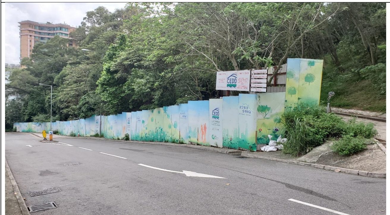
Photo 2 - Existing Slope to the South of the Proposed Ancillary Building Currently under Landslip Prevention and Mitigation Works
