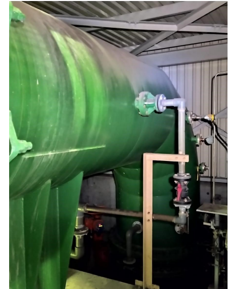
Photo 19: Circulating Water Pipe emerging from underground
