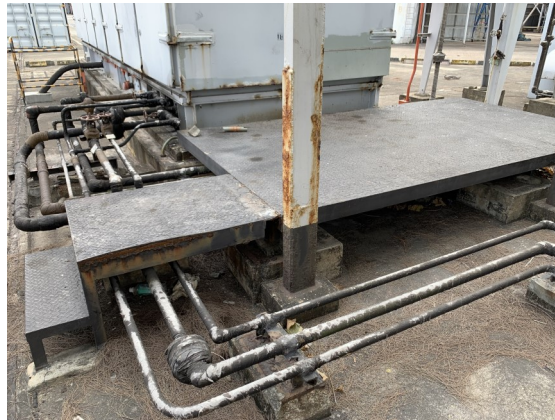
Photo 11: Diesel supply pipes
