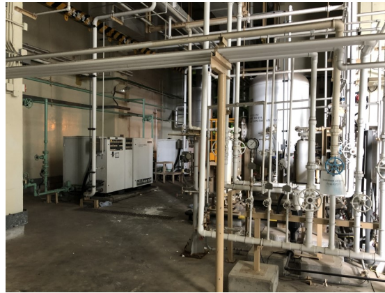
Photo 14: Gas tanks installed at the ground floor of GT57 Auxiliary Building
