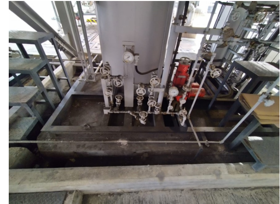
Photo 15: Chemical Dosing Pit (Hydrazine Hydrate Tank) at the ground floor of GT57 Auxiliary Building
