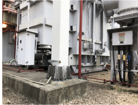
Photo 8: GT's transformer concrete bund filled with pebbles
