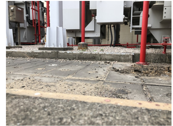
Photo 9: GT's transformer concrete paved ground
