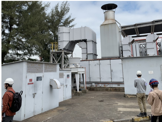
Photo 10: Black Start Generator set (one (1) diesel generator and three (3) air compressor units).
