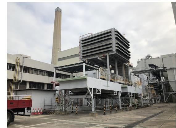
Photo 6: Gas Turbine Unit 7
