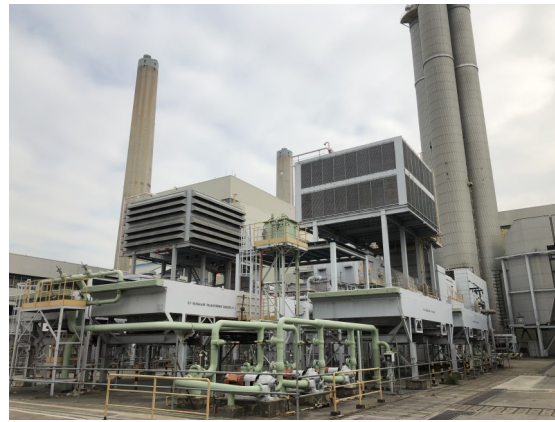
Photo 5: Gas Turbine Unit 6
