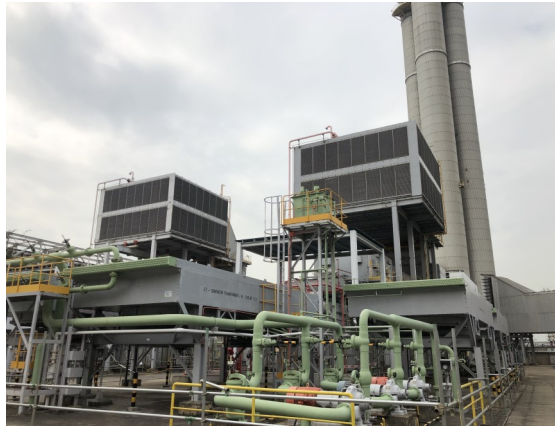
Photo 2: Gas Turbine Unit 3
