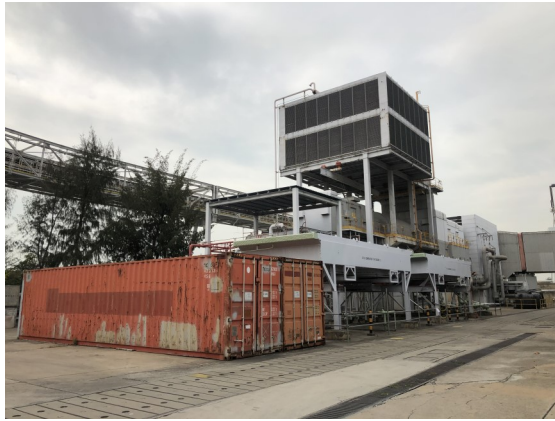
Photo 1: Gas Turbine Unit 2
