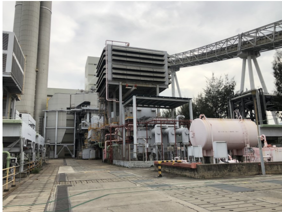
Photo 4: Gas Turbine Unit 5
