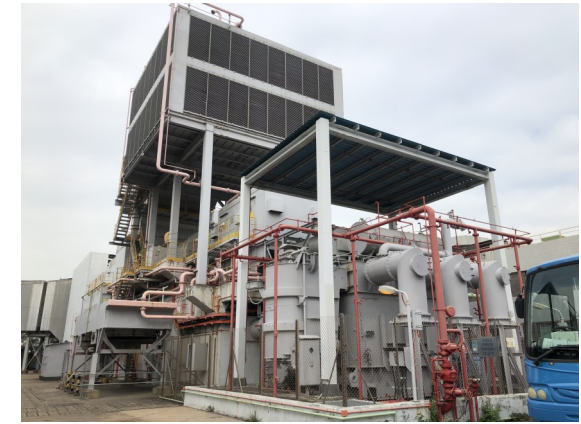
Photo 3: Gas Turbine Unit 4
