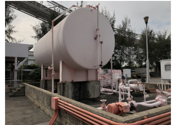
Photo 12: Lube oil tank
