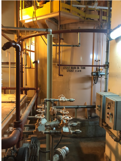
Photo 16: Main oil tank installed at the ground floor of GT57 Auxiliary Building
