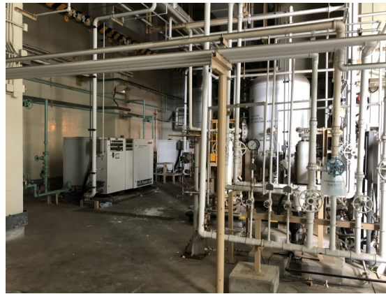
Photo 14: Gas tanks installed at the ground floor of GT57 Auxiliary Building
