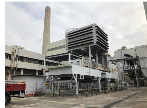
Photo 6: Gas Turbine Unit 7
