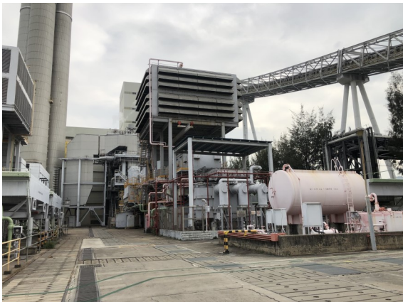
Photo 4: Gas Turbine Unit 5
