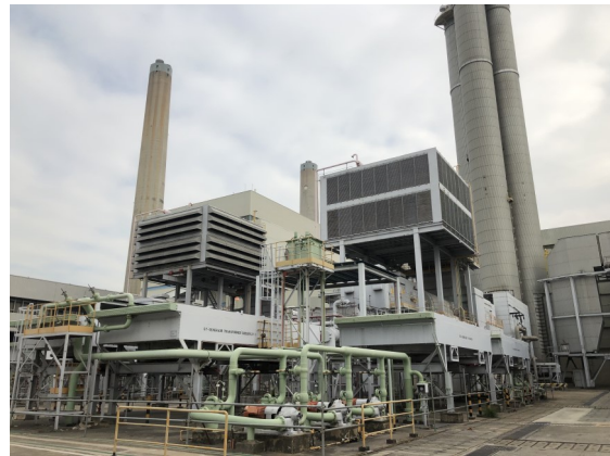
Photo 5: Gas Turbine Unit 6
