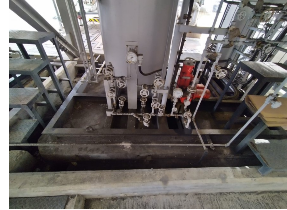
Photo 15: Chemical Dosing Pit (Hydrazine Hydrate Tank) at the ground floor of GT57 Auxiliary Building
