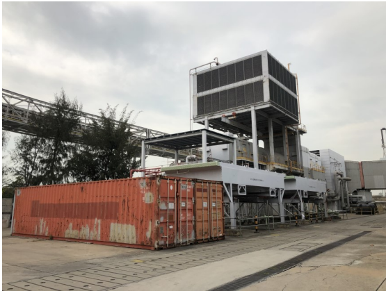
Photo 1: Gas Turbine Unit 2
