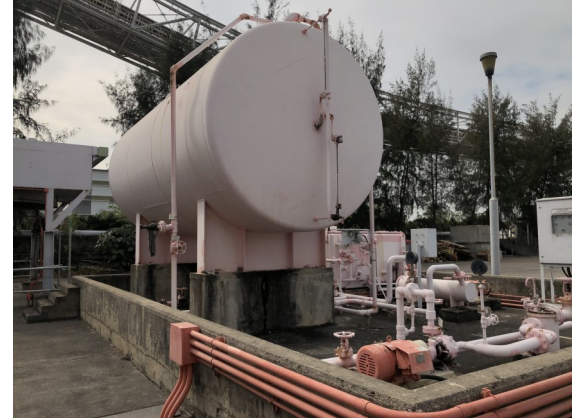
Photo 12: Lube oil tank
