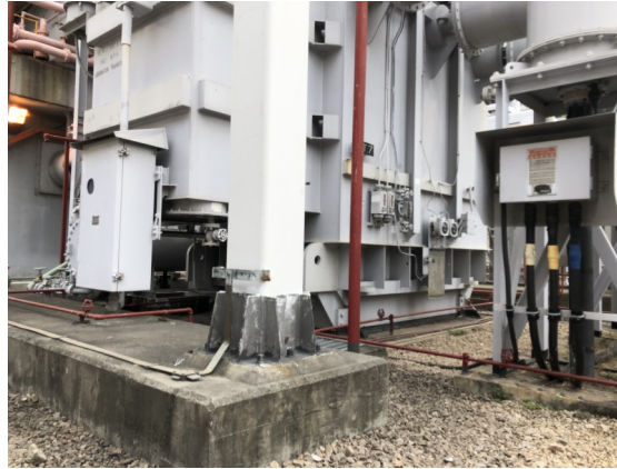
Photo 8: GT's transformer concrete bund filled with pebbles
