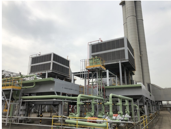
Photo 2: Gas Turbine Unit 3
