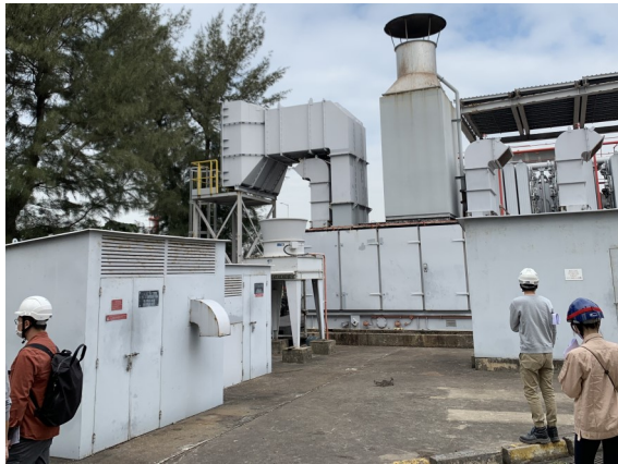
Photo 10: Black Start Generator set (one (1) diesel generator and three (3) air compressor units).
