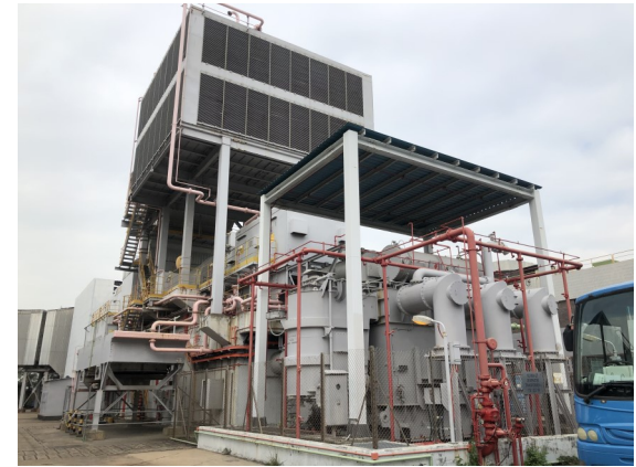
Photo 3: Gas Turbine Unit 4
