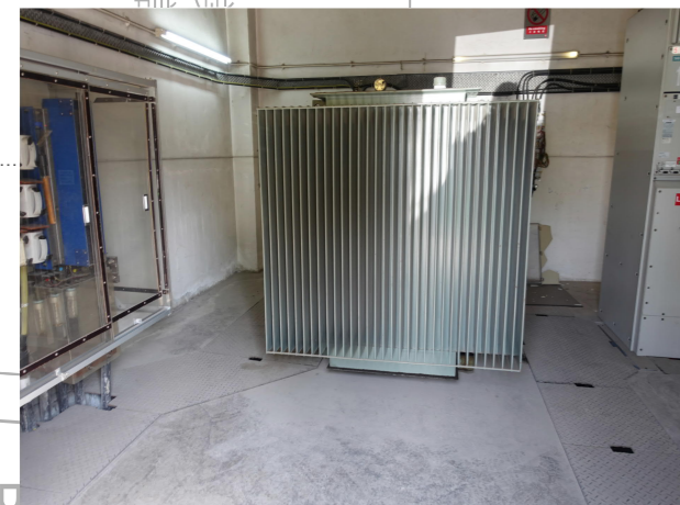
PHOTO 5894: TRANSFORMER IN ELECTRICAL SUBSTATION IN TUEN MUN SWIMMING POOL (SITE TME-S3) (DATE TAKEN: 4 FEBRUARY 2021)
