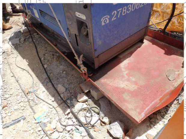
PHOTO 2624: GENERATOR (SITE TME-S4) AND GROUND CONDITION AROUND WORKS AREA OF CONTRACT NO. DC/2018/09 (DATE TAKEN: 21 MAY 2021)
