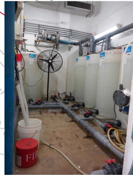
PHOTO 4705: STORAGE ROOM OF SODIUM HYPOCHLORITE (BLEACH) (DATE TAKEN: 25 JANUARY 2021)
