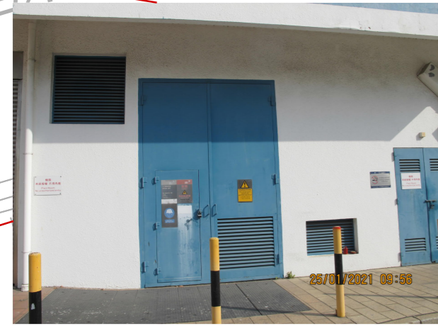
PHOTO 0858: ELECTRICAL SUBSTATION IN TUEN MUN SWIMMING POOL (SITE TME-S3) (DATE TAKEN: 25 JANUARY 2021)
