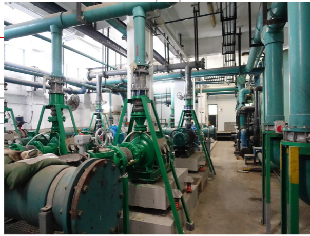
PHOTO 4655: PLANT ROOM (DATE TAKEN: 25 JANUARY 2021)
