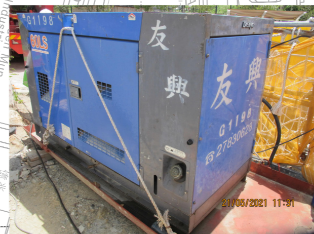
PHOTO 7461: GENERATOR AT WORKS SITE OF CONTRACT NO. DC/2018/09 (SITE TME-S4) (DATE TAKEN: 21 MAY 2021)
