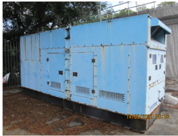
PHOTO 7329: EXISTING BACKUP GENERATOR (DATE TAKEN: 14 MAY 2021)
