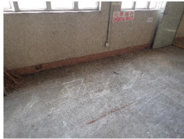
PHOTO 2191: FORMER CHEMICAL WASTE STORAGE AREA IN FORMER WORKSHOP IN ADMINISTRATION BUILDING (DATE TAKEN: 14 MAY 2021)
