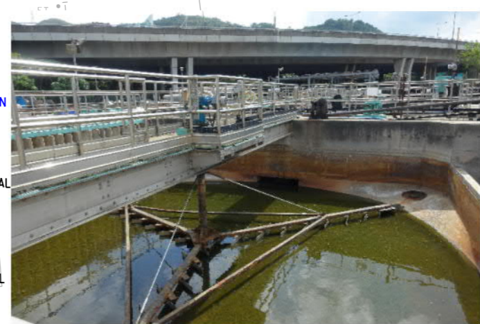
PHOTO 6870: DISUSED DETRITOR (DATE TAKEN: 14 MAY 2021)
