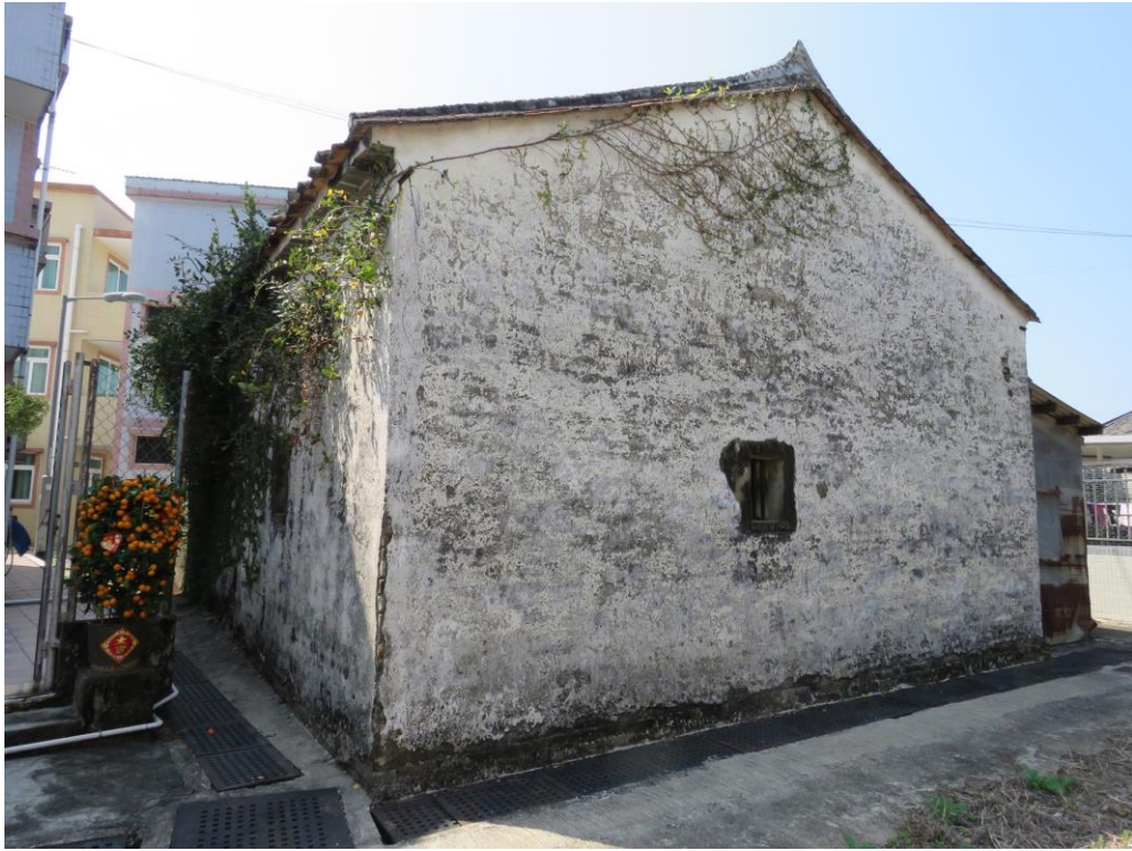
Side and back view of HB-21, showing northeast and southeast elevations, looking west.
