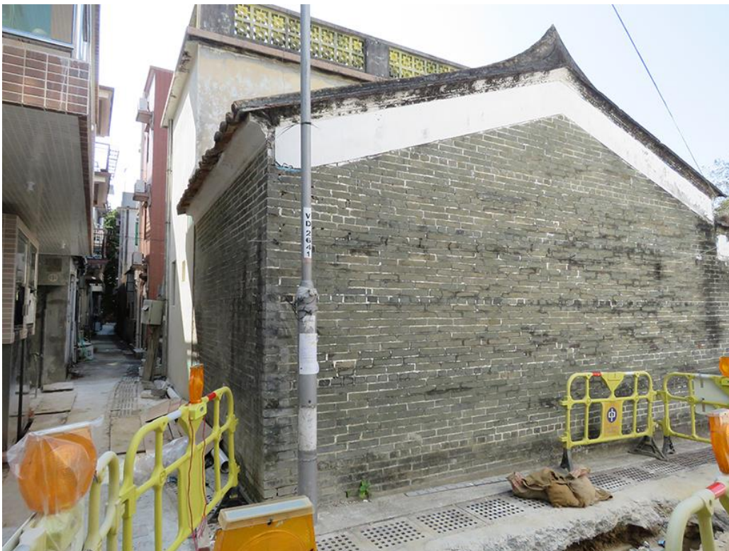
Back and side view, HB-33, showing south and east elevations, looking northwest.
