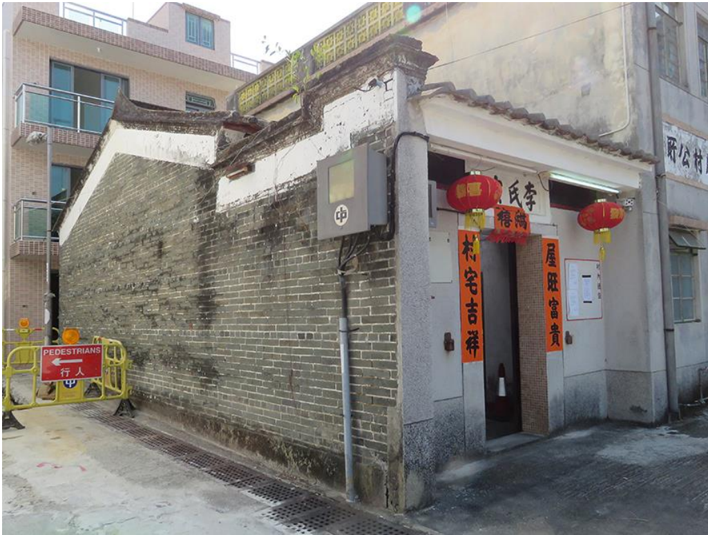
Side and front view of HB-33, showing east elevation and façade, looking southwest.
