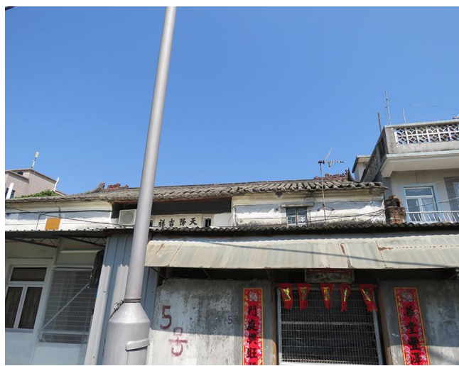
Façade of No.4 and 5 blocked by temporary structures in front, looking northeast.
