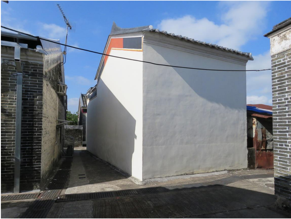
Side and back view of GB-04, showing southwest and southeast elevations, looking north.
