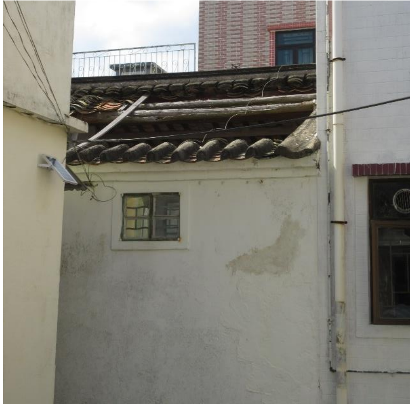
Rear of No.26A with view of collapsed roof
