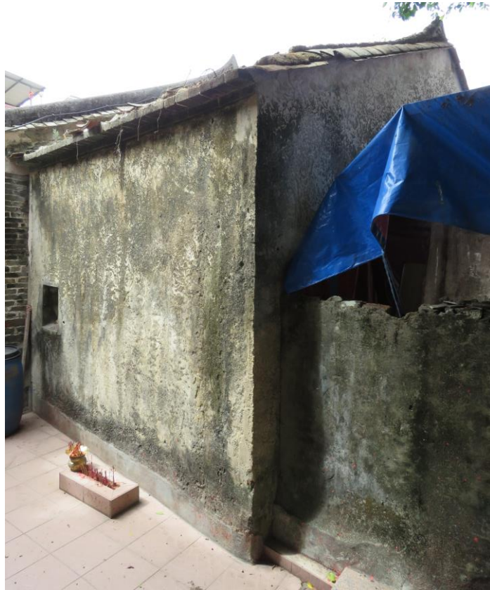
Back and side view of HB-48, showing southeast and northeast elevations, looking southwest.
