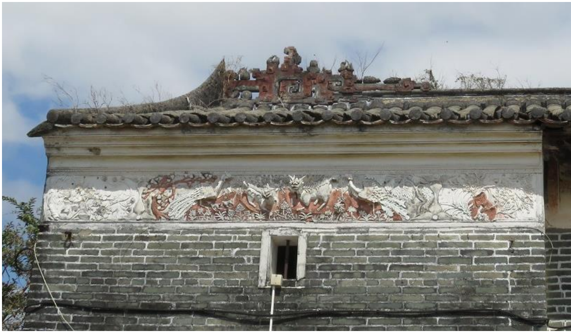
Relief carving and decorative geometric plaster mouldings on roof ridge of No.138
