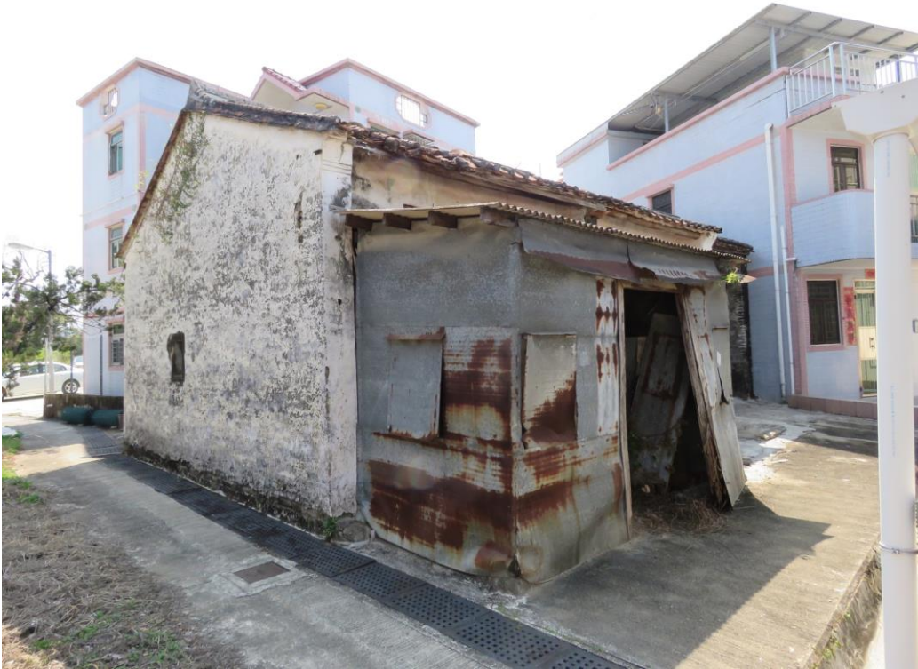
General view of HB-21, showing northeast elevation and the front, looking southwest.
