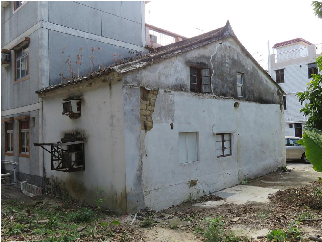
Back and side view of HB-65, showing northeast and northwest elevations, looking southwest.
