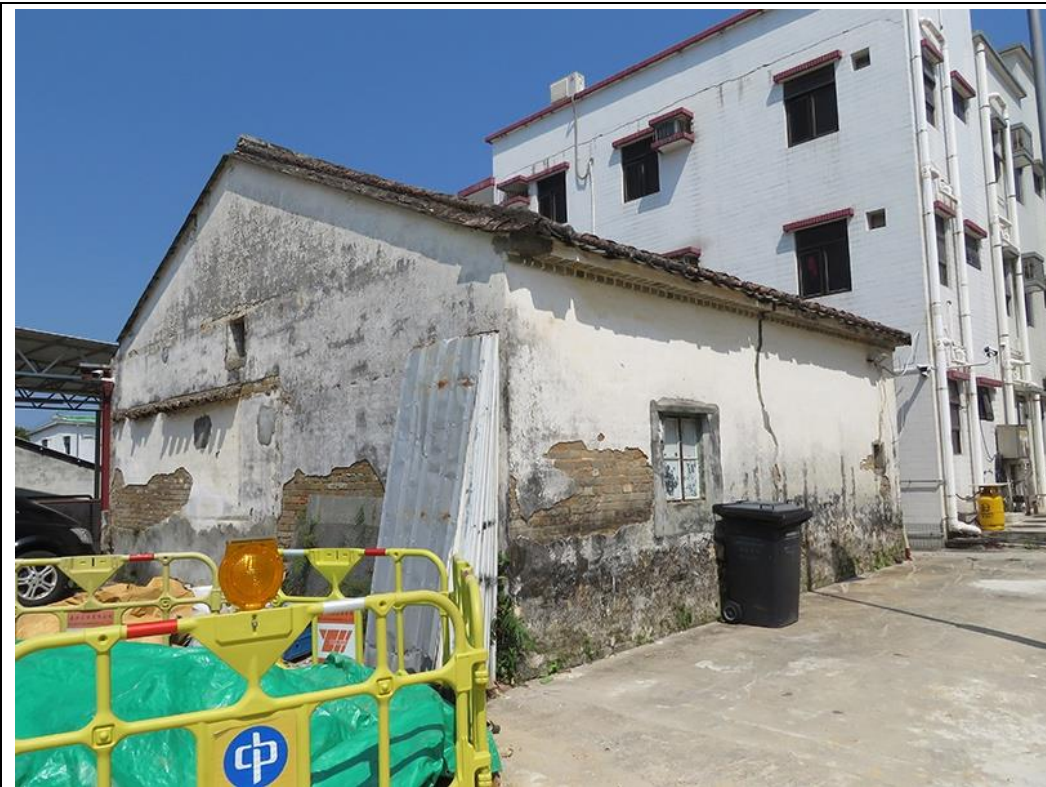
Side and back view of HB-22, showing southwest and southeast elevations, looking northeast.
