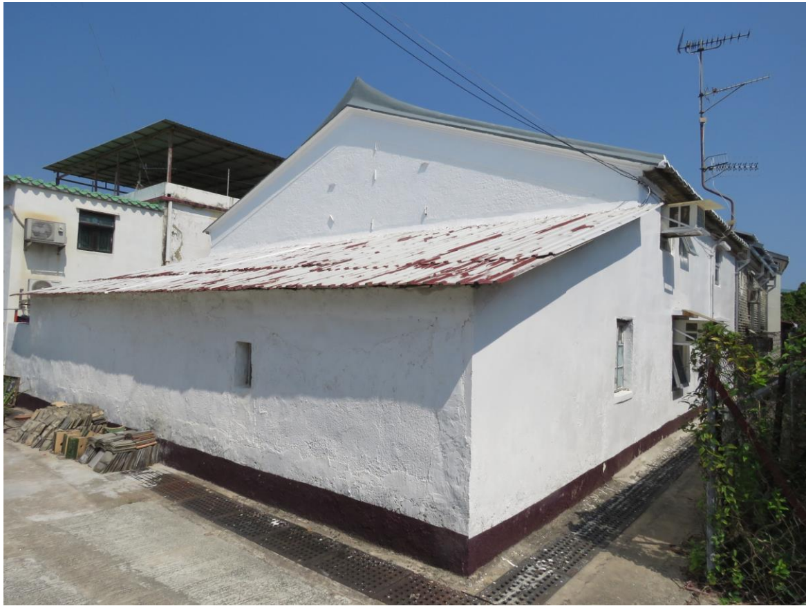
Side and back view of HB-17, showing southwest and southeast elevations, looking northeast.
