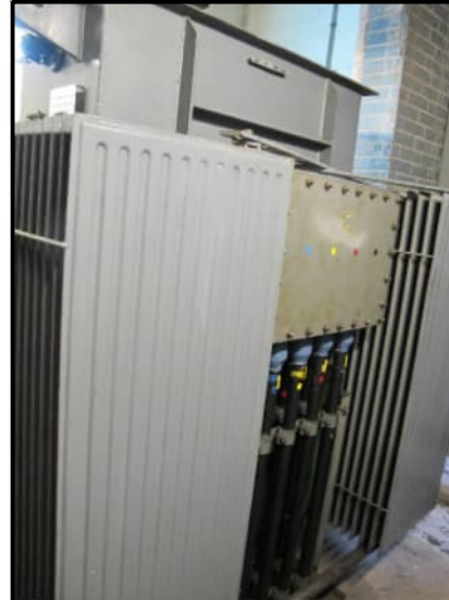
PHOTO 9882: TRANSFORMER K1-2 IN VENTILATION BUILDING K1 (DATE TAKEN: 25 AUGUST 2020)
