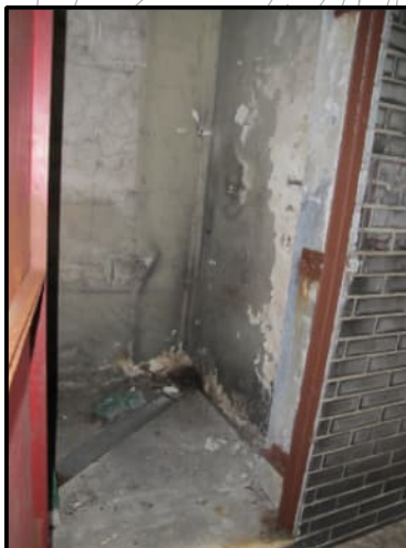
PHOTO 9872: CHEMICAL WASTE STORAGE AREA IN VENTILATION BUILDING K2 (DATE TAKEN: 25 AUGUST 2020)
