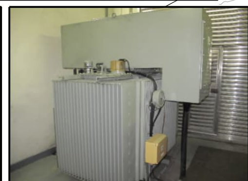
PHOTO 9867: TRANSFORMER K2 IN VENTILATION BUILDING K2 (DATE TAKEN: 25 AUGUST 2020)
