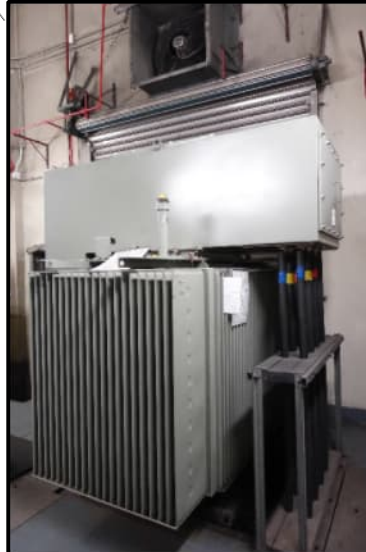
PHOTO 2881: TRANSFORMER K1 IN VENTILATION BUILDING K1 (DATE TAKEN: 25 AUGUST 2020)
