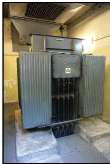
PHOTO 2752: TRANSFORMER S1-2 IN S1-2 BUILDING (DATE TAKEN: 25 AUGUST 2020)
