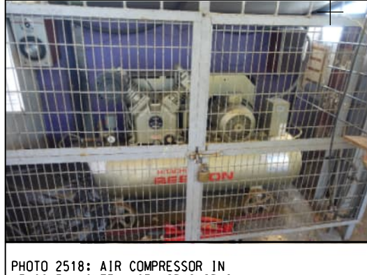
PHOTO 2518: AIR COMPRESSOR IN VEHICLE MAINTENANCE WORKSHOP IN ADMINISTRATION BUILDING (DATE TAKEN: 25 AUGUST 2020)
