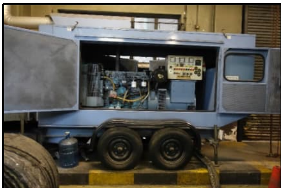
PHOTO 2835: MOBILE GENSET 1 IN VENTILATION BUILDING K2 (DATE TAKEN: 25 AUGUST 2020)
