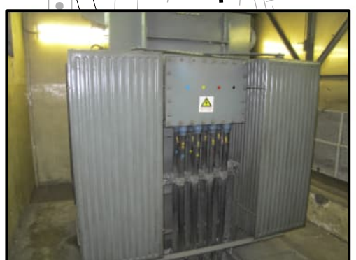
PHOTO 9857: TRANSFORMER K2-2 IN K2-2 BUILDING (DATE TAKEN: 25 AUGUST 2020)
