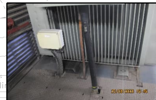
PHOTO 4462: TRANSFORMER K1-2 IN VENTILATION BUILDING K1 (DATE TAKEN: 25 AUGUST 2020)
