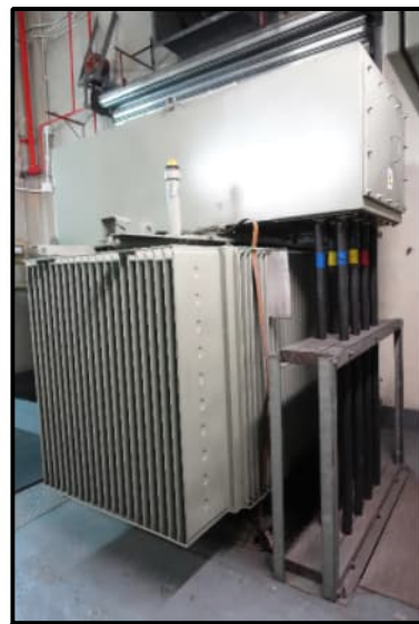
PHOTO 2783: TRANSFORMER S1 IN VENTILATION BUILDING S1 (DATE TAKEN: 25 AUGUST 2020)
