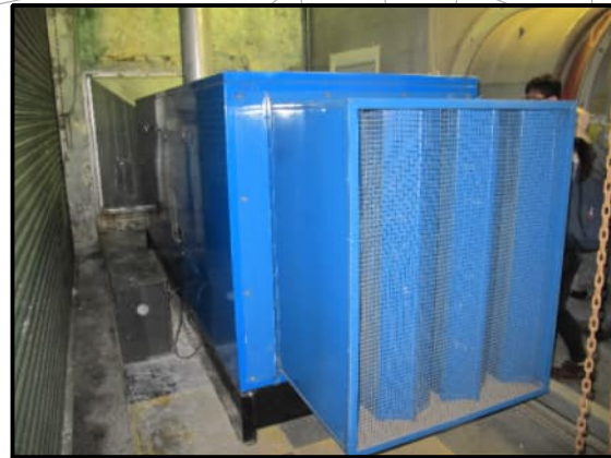
PHOTO 9838: GENERATOR S1 IN VENTILATION BUILDING S1 (DATE TAKEN: 25 AUGUST 2020)
