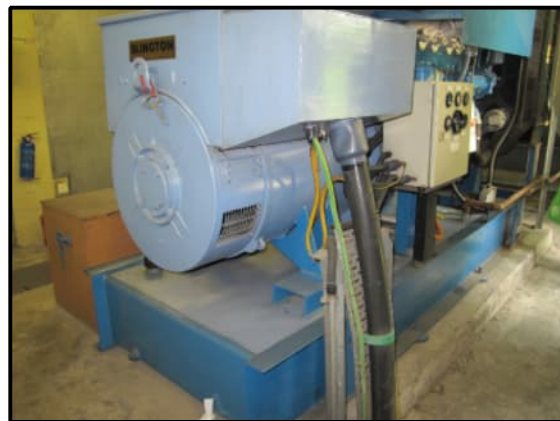
PHOTO 9827: GENERATOR S1-2 IN S1-2 BUILDING (DATE TAKEN: 25 AUGUST 2020)
