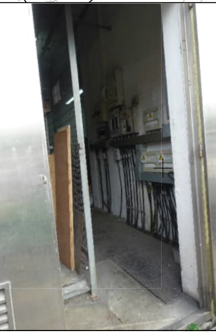
PHOTO 2725: SWITCH ROOM IN E&M BUILDING (DATE TAKEN: 25 AUGUST 2020)
