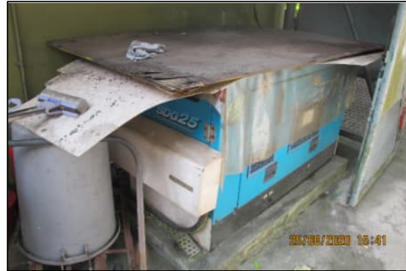
PHOTO 4378: GENERATOR (DATE TAKEN: 25 AUGUST 2020)
