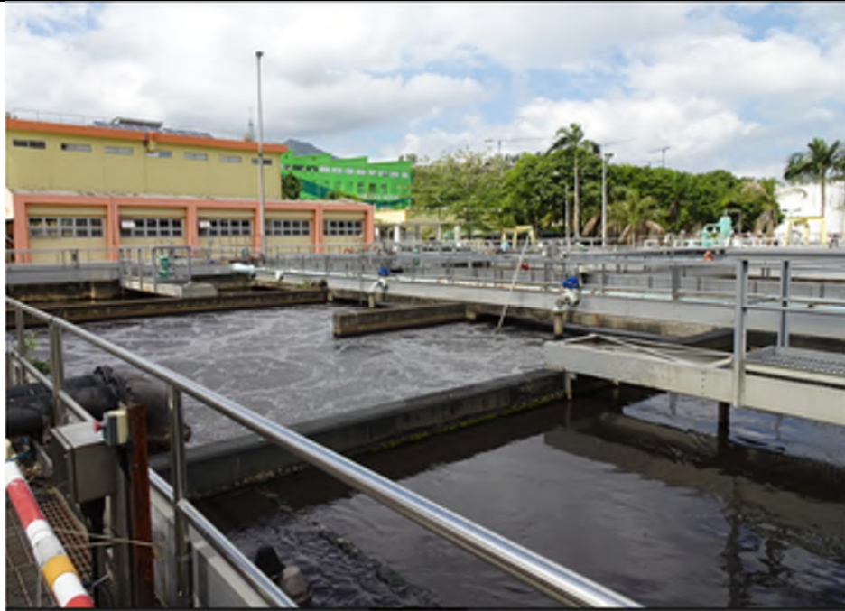
Photo WP-36: Aeration Tanks of West Plant - The tanks are located on concrete paved floor in good condition with no oil stain/stressed vegetation observed.
