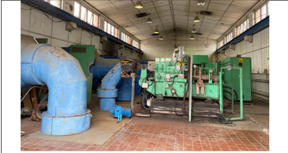
Photo WPS-7: Blower House (Air Blowers on Ground Floor) – The air blowers are located on ceramic tiles and concrete paved floor in good condition with no oil stain observed.
