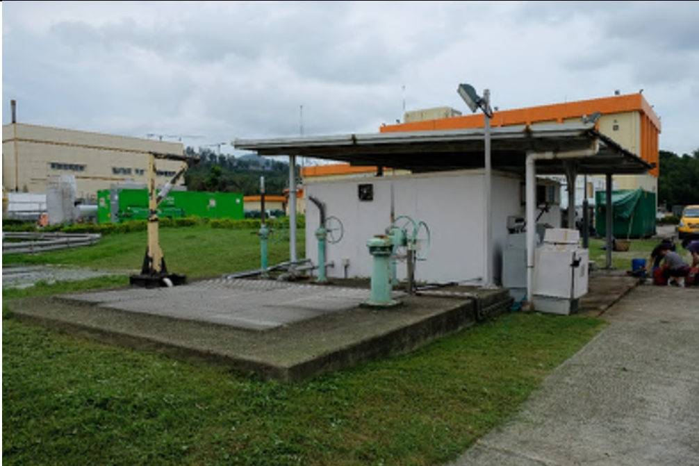
Photo WPS-36: Effluent Sampling shelter – Effluent sampling equipment is observed in this location. The facility is surrounded by vegetation and concrete paved surface. No sign of land contamination such as oil stains is identified.
