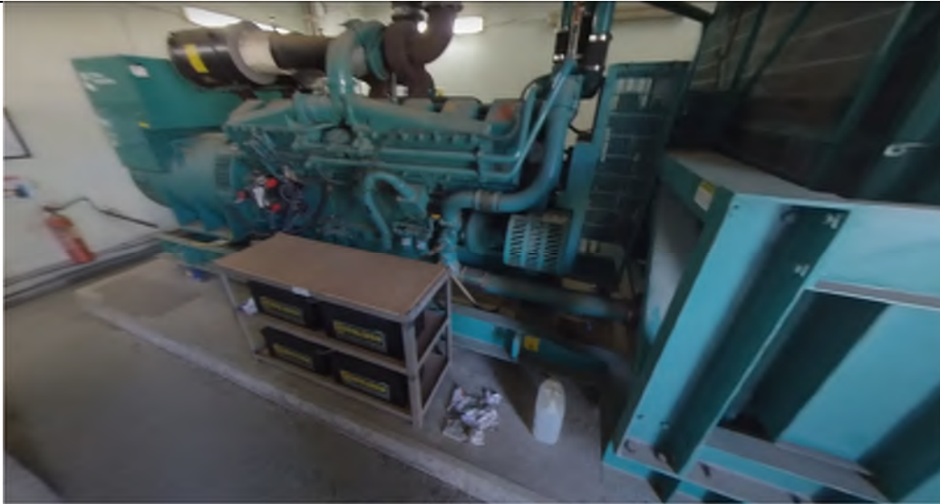
Photo EP-40:Screen House –Emergency generators are located within the Screen House. The floor is paved with concrete slab next to the Generator Daily Fuel Tank on elevated concrete paved platform. No oil stain/leakage is observed in this located.
