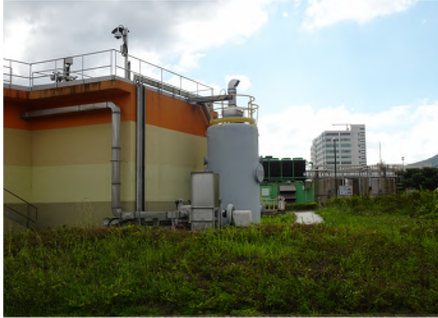
Photo EP-21: Decanting Chamber – The chamber is located on concrete paved floor connecting to the Primary Sludge Gravity Thickener surrounding by vegetation. There is no stressed vegetation/ leakage is observed. The chamber is in good condition where no damage or large area of dirty stain is found.
