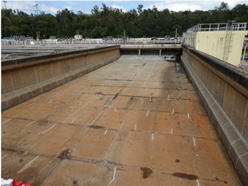
Photo V8: Primary Sedimentation Tanks of East Plant – A tank was under maintenance. The tank is constructed with concrete. No observation of damage/ leakage is observed. Only water stain and stain caused by years of functioning is observed.
