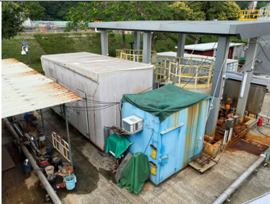
Photo EP-10: Ferric Chloride Dosing System #2 (to the north of sludge Consolidation Tanks in East Plant) – This system is located on concrete paved floor. water stain and rusty stain were observed due to weathering and cleaning activities. Shelter is built to protect facility from being damaged by extreme weather.
