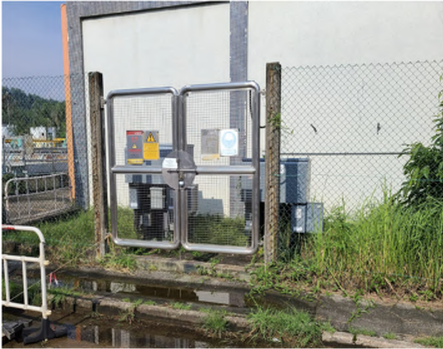
Photo WPS-35: Transformer – The transformer is located on concrete paved floor surrounded by vegetation. Cracks are observed near the transformer. However, the transformer is in good condition and maintained by CLP no leakage of transformer oil is observed. No oil stain/leakage is found in this location.
