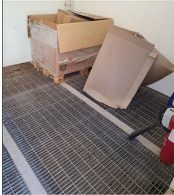
Photo EP-42: Chemical Store – Leatheroid are found on steel panel inside the chemical store above concrete paved floor. Some leatheroid are located on wooden panel. No oil stain/leakage is observed.
