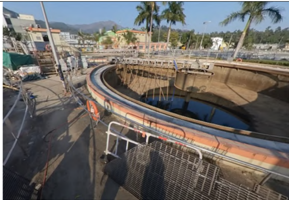
Photo WP-38: Primary Sedimentation Tanks of West Plant – The tanks are located on concrete paved floor in good condition with no oil stain/stressed vegetation observed.
