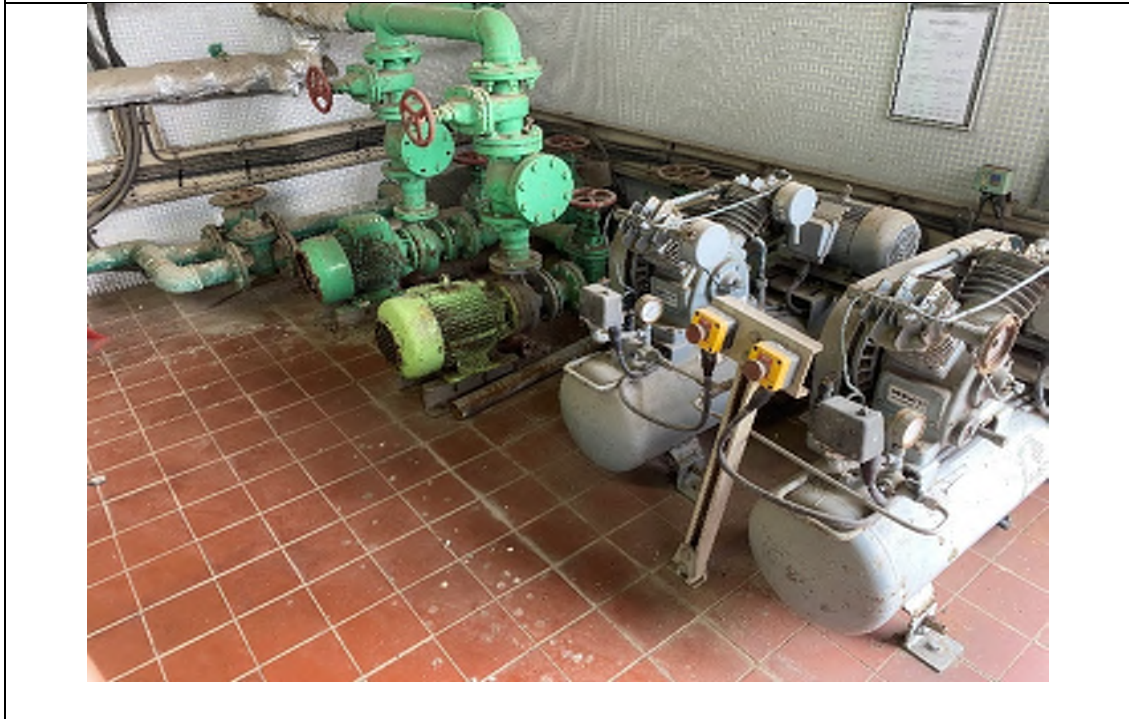
Photo WPS-8: Blower House (Pumps on Ground Floor) – Pumps are located on ceramic tiles and concrete paved floor in good condition with no oil stain observed.
