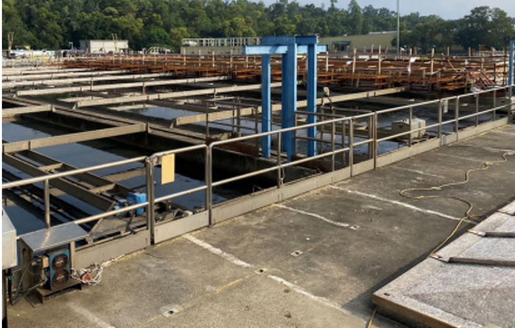
Photo V6: Primary Sedimentation Tanks of East Plant – The tanks are constructed with concrete on a raised slope. Only stain caused by weathering is observed, no oil stain/ leakage is observed in the area.
