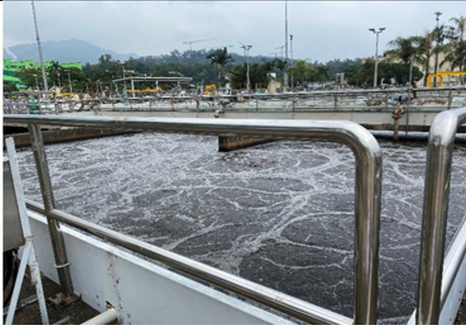
Photo WP-35: Aeration Tanks of West Plant – The tanks are located on concrete paved floor in good condition with no oil stain/stressed vegetation observed.
