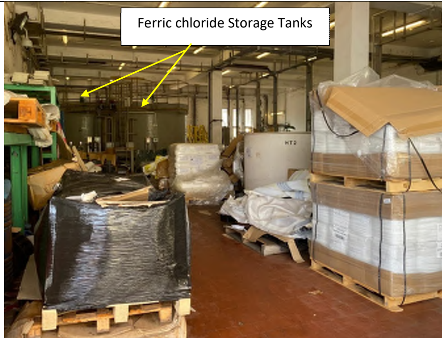
Photo WPS-17: Chemical House – Equipment are stored and placed on wood panel inside the Chemical House with ceramic tiles with concrete paved floor. Only Ferric Chloride Storage Tanks were observed at this location, no other chemicals are stored at Chemical House. No oil stain is observed
