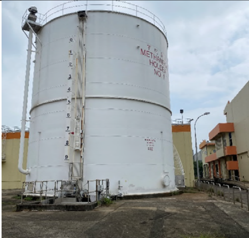
Photo WPS-9: Bio-Gas Holding Tank of West Plant– The Bio-Gas Holding Tank is located on concrete paved floor in good condition with no oil stain observed.
