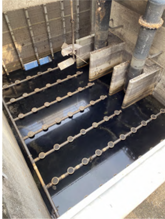
Photo V10: Aeration Tanks of East Plant– The tanks are constructed with concrete, no broken or damage is observed. Just stain caused by weathering is observed.
