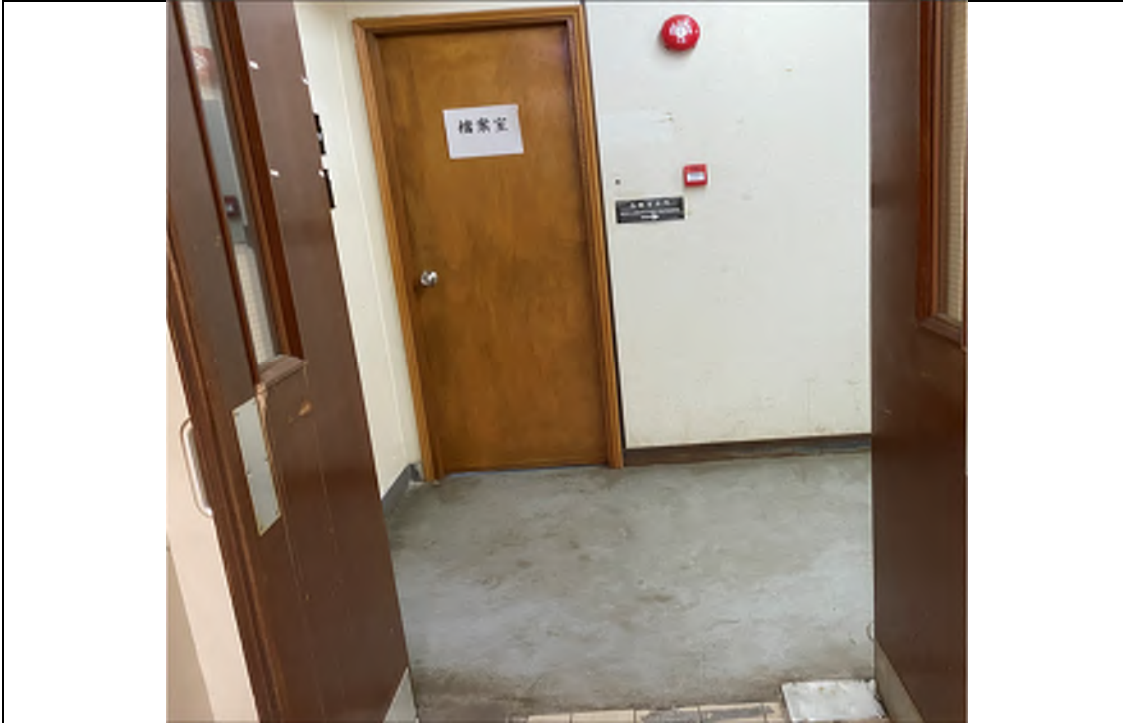
Photo WP-15: Administrative Building (Second Floor) – The Document Room is located on concrete paved floor opposite to the laboratory. No oil stain/ leakage is observed.
