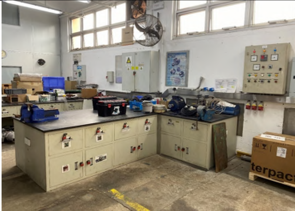
Photo WP-5: Electrical Workshop - The tool desks are located on concrete paved floor with small area of water stain is observed. Maintenance work of small equipment was carried out. Cracks were observed on the floor. No oil stain / leakage is observed.
