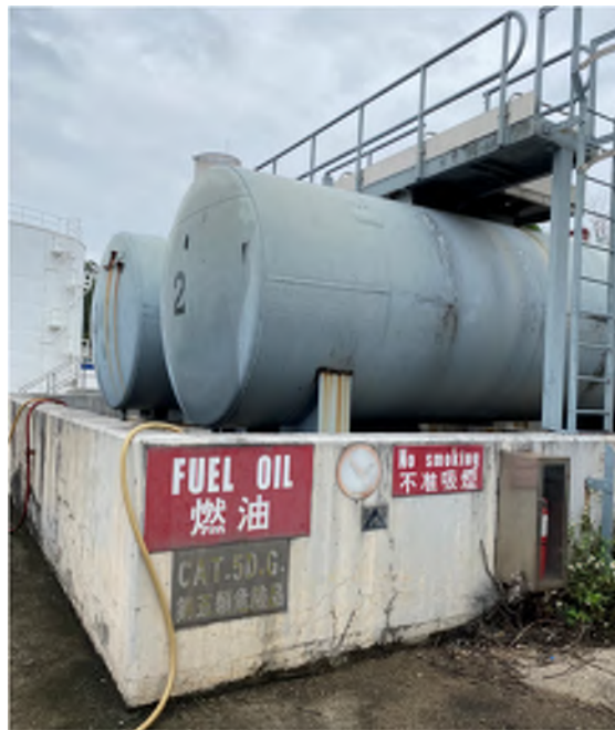
Photo EP-29: Waste Bio-Gas Burner – The burner is located on an elevated platform with concrete slab on concrete paved floor. Fuel oil tanks are within bunded area and protected by concrete slab. No oil stain/ leakage is observed.
