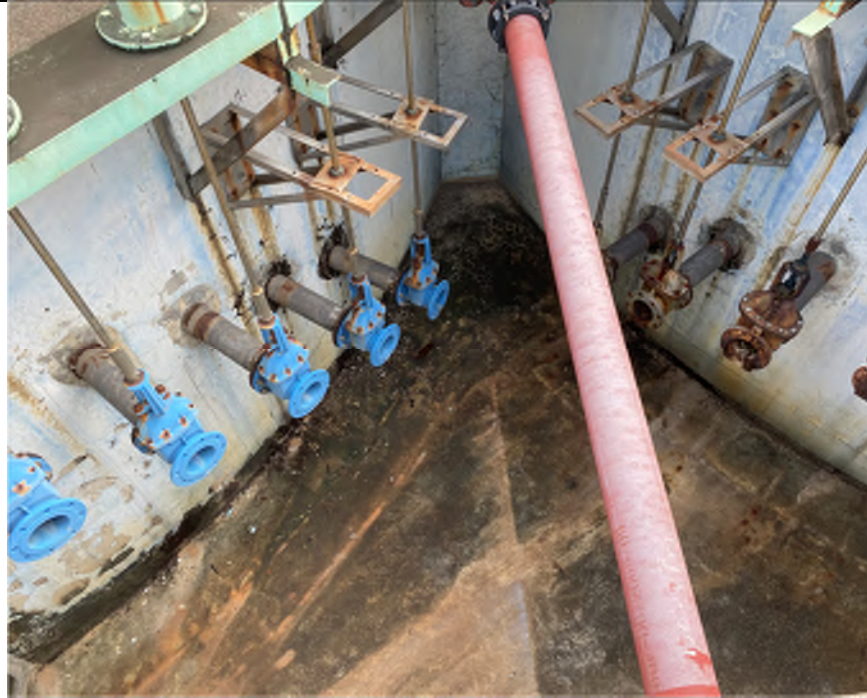
Photo EP-9: Sludge Consolidation Tanks of East Plant (Ground Floor) - The floor is paved with concrete, dirty stain and water stain caused by weathering and handling of sludge is observed. There is no damage or broken tools observed.
