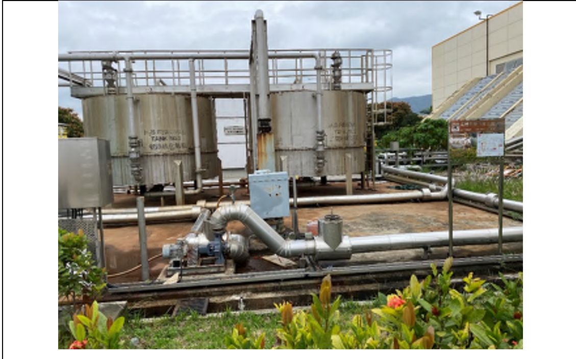
Photo EP-25: Combined Heat and Power Generating System of East Plant – The system is located on concrete paved floor with vegetation surrounding. No stressed vegetation is observed and the system is in good condition with no damage observed. No oil stain/leakage is observed in the area. Rusty stain is observed in this location.
