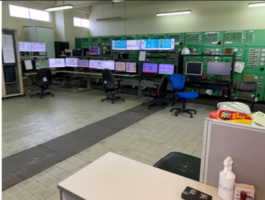
Photo WP-20: Control and Storage House (Control Room with Control Panels on Second Floor) - The floor is paved with ceramic tile and concrete in good condition. No oil stain/leakage is observed.
