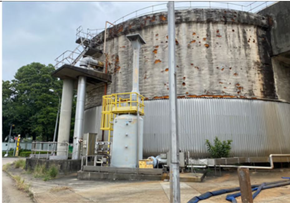
Photo WPS-10: Sludge Digestion Tank of West Plant – The tank is located on concrete paved floor in good condition with no oil stain/stressed vegetation observed.
