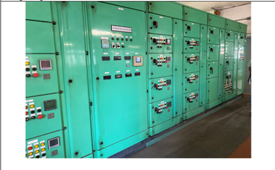
Photo WPS-4: Sludge Pumping Station – The Control Panel is located above the basement level with concrete paved floor in good condition with no oil stain observed.
