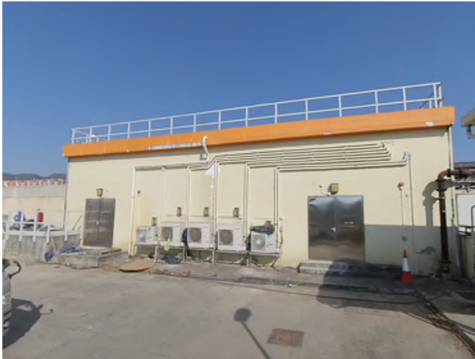
Photo V11 : Switch Room – The Switch Room is located on concrete paved floor, it is a one-storey building. No oil stain/leakage is observed.
