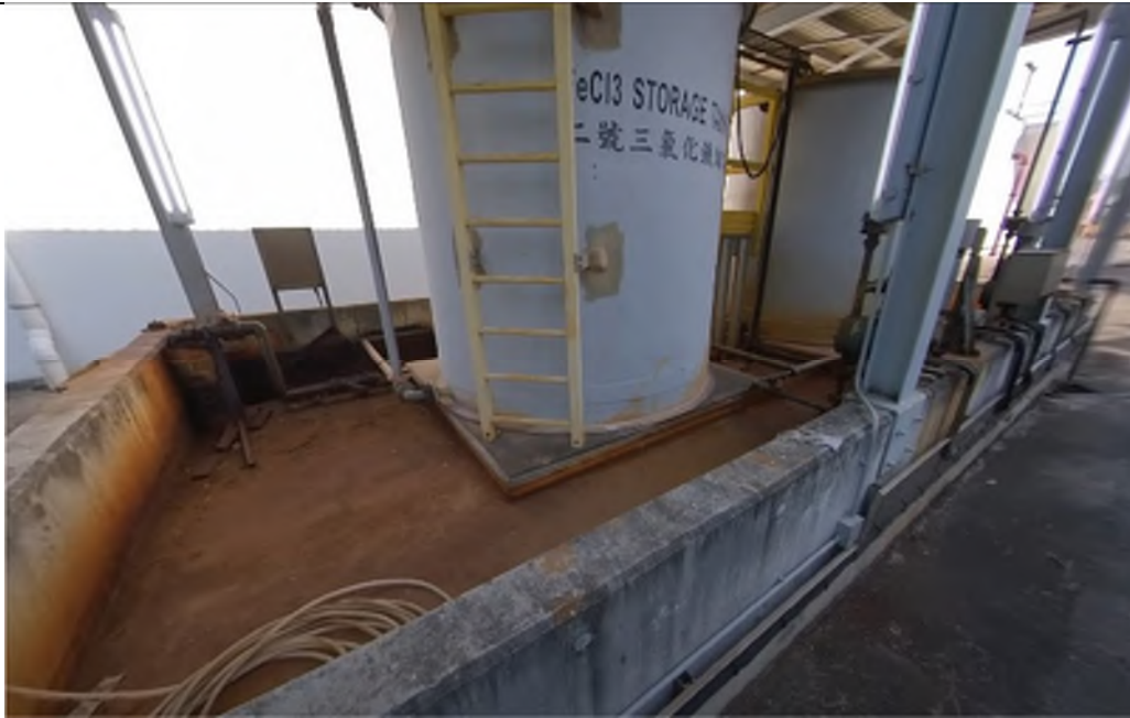
Photo WPS-27 :Ferric Chloride Dosing System #1 - The system is located on an elevated platform with concrete slab. Two FeCl3 Storage Tanks are located under the shelter.
