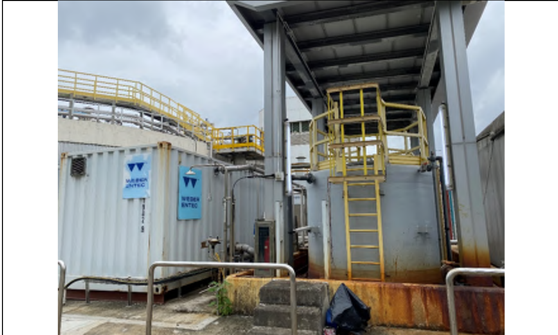
Photo EP-13: Ferric Chloride Dosing System #2 – The system is located on an elevated platform with concrete slab. Two FeCl 3 Storage Tanks are located under the shelter. Ferric Chloride stain is observed.
