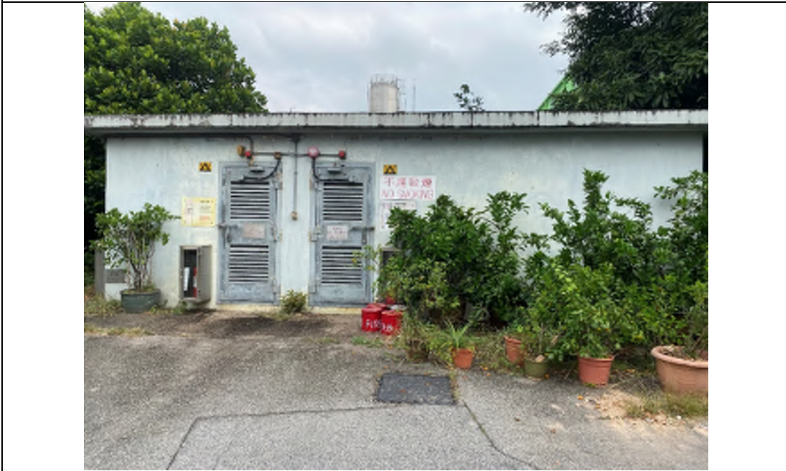
Photo WP-22: Dangerous Goods (DG) Store (External View) - The DG Store is located on concrete paved floor. No oil stain/ leakage is observed.
