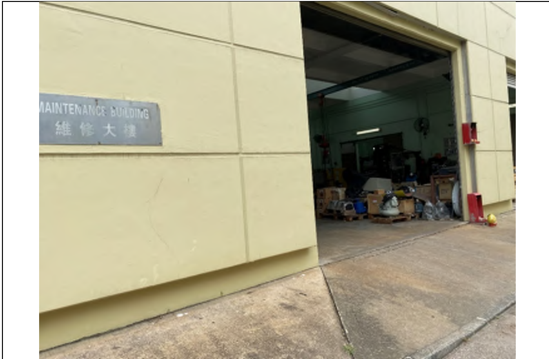
Photo WP-9: Maintenance Building (External View) – The building is located on concrete paved floor, stain caused by weathering can be observed. No oil stain / leakage is observed.
