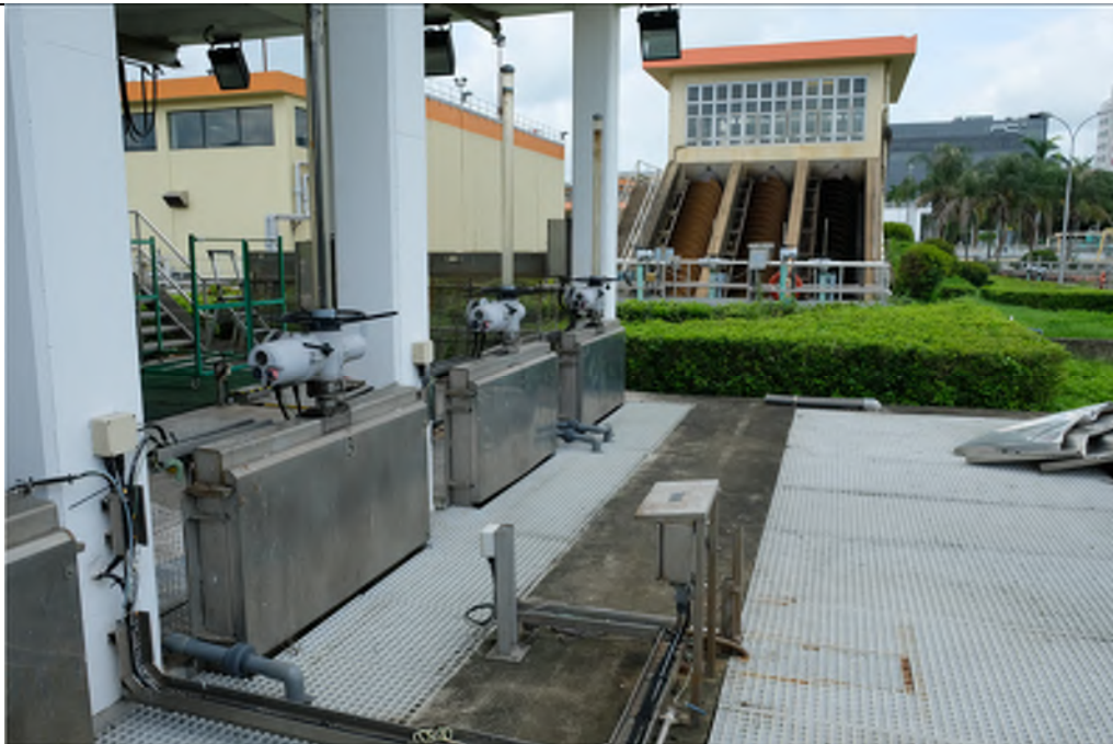
Photo WPS-28: UV Disinfection Facilities – The UV Disinfection Facilities is located on concrete paved slab. Vegetation is observed near the facilities in good condition. No oil stain/ leakage is observed.
