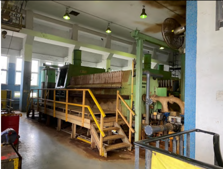
Photo WPS-20: Sludge Dewatering House (Upper Floor) – The upper floor is paved with concrete in good condition. The area is clean and dry with no oil stain.
