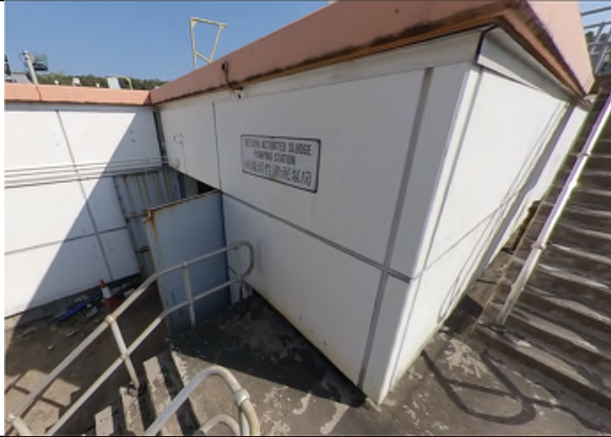
Photo V12: Return Activated Sludge Pumping Station – The Station is located on floor paved with concrete, stain caused by weathering is observed. No oil stain/leakage is observed.
