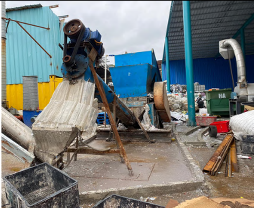
Photo EA-38: Lot No. STT 1745 - Existing Lau Choi Kee Plastic Company Limited – The waste water pumping machine was located outside the warehouse and shelters. Concrete made barriers were observed surrounding the machine on the floor to prevent water from leaking out. Dirty stain and debris were observed with no oil stain/leakage was observed.
