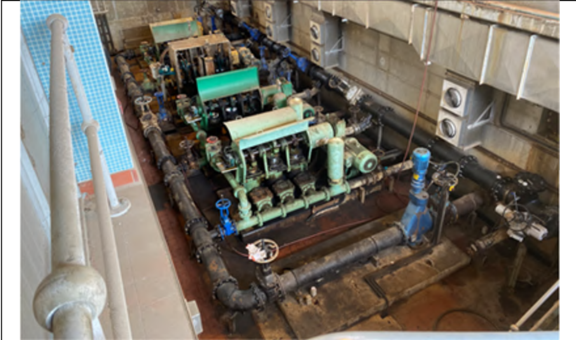
Photo WPS-3: Sludge Pumping Station (Below Ground Level) - The Sludge Pumps are located on concrete floor in good condition with no oil stain. The stains observed were stains of sewage sludge.
