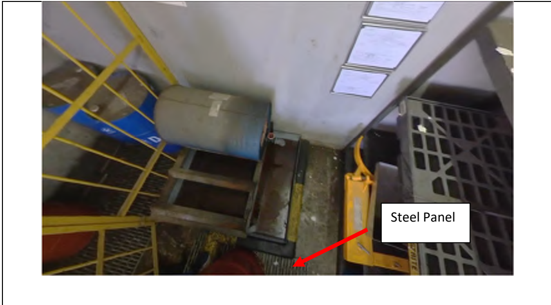
Photo EP-24: Lubricant Oil Store (Lubricant Oil Storage Room) – The floor of the room is paved with concrete and steel panel. Oil stain and leakage is observed on the floor of the storage room. Spillage is observed during the site walk. Potential land contamination issue is anticipated.
