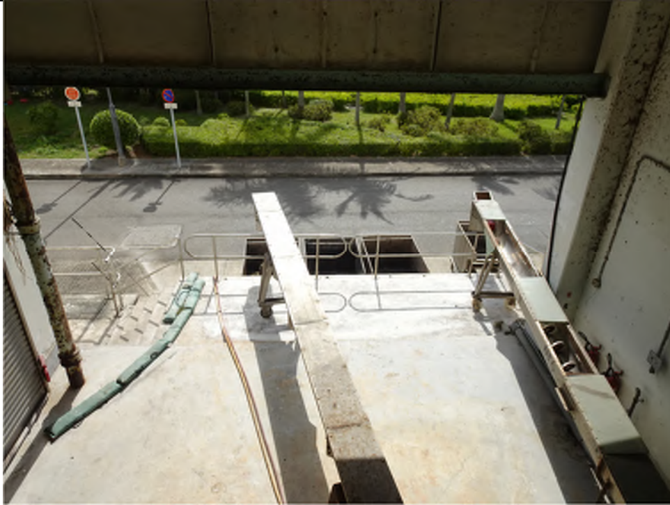
Photo EP-17: Screen House – The first floor of the screen house is located above ground level with concrete paved floor in good condition, no stain is observed.
