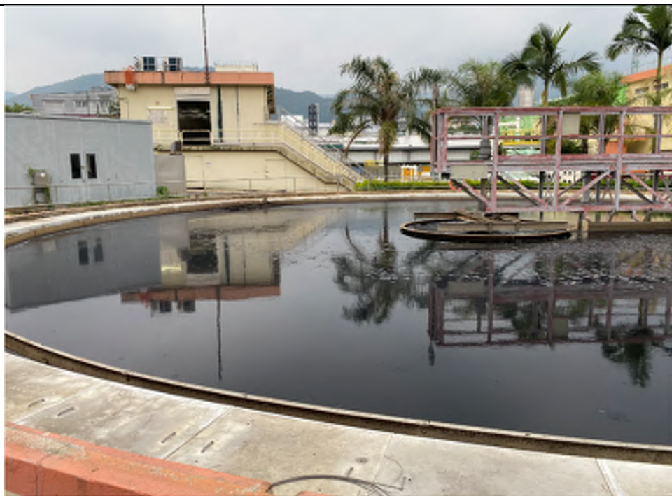
Photo WP-34: Primary Sedimentation Tanks of West Plant - The tanks are located on concrete paved floor in good condition with no oil stain/stressed vegetation observed.
