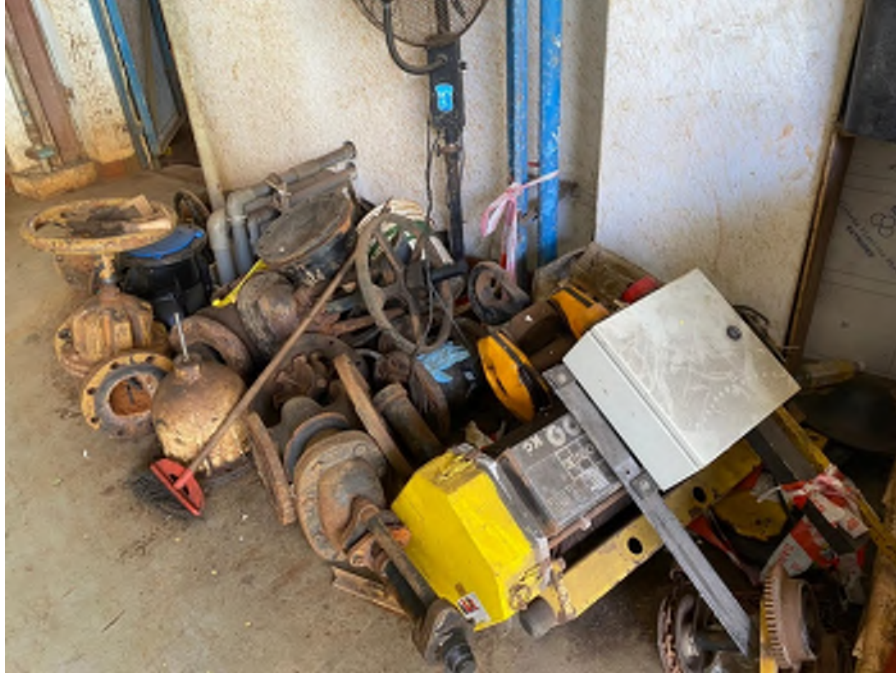
Photo WPS-19: Chemical House – Some tools and equipment are placed on concrete paved floor, no oil stain is observed. No storage of COC is recorded / observed.
