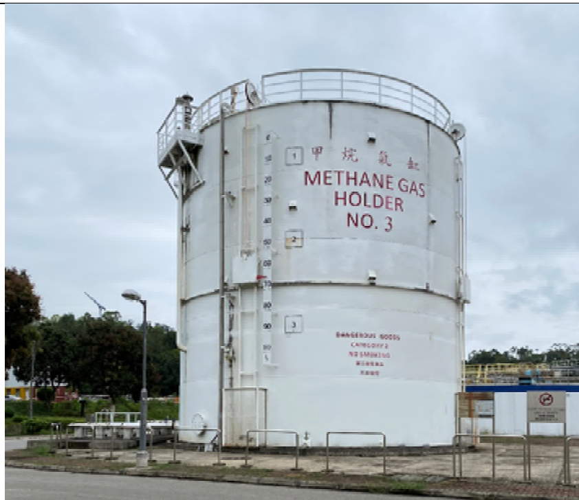
Photo EP-14: Bio-gas Holding Tank #1 (to the west of Sludge Consolidation Tanks) in East Plant - The tank is located on concrete paved floor with no stressed vegetation/ leakage is observed. The tank is in good condition no damage/ leakage is observed.
