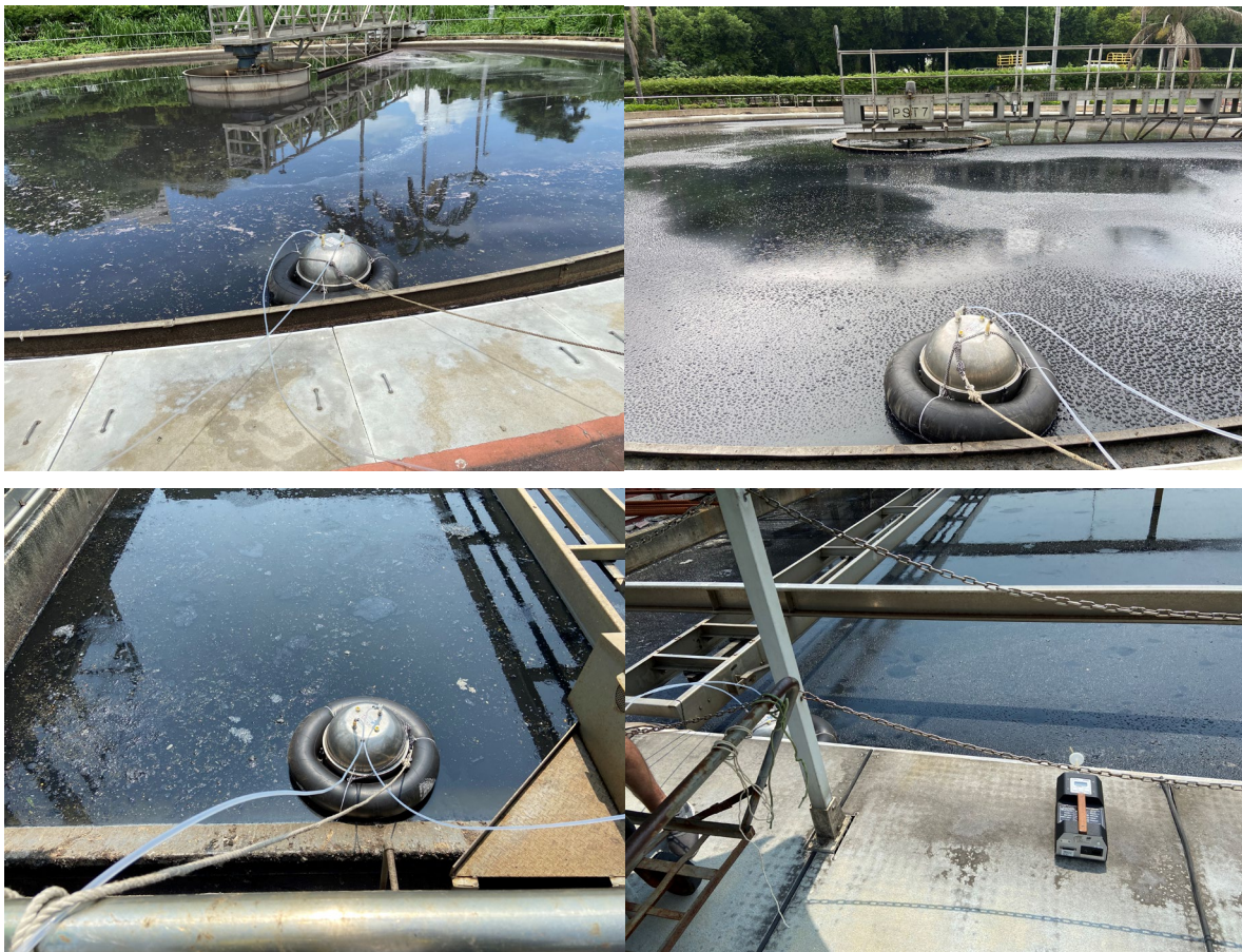
Figure 9.3 Photos of the west and east sedimentation tanks at TPSTW
