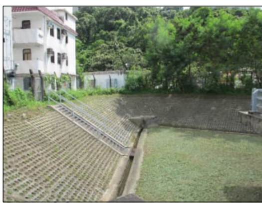
PHOTO 9507: POLDER OF FO TAN NULLAH (DATE TAKEN: 14 AUGUST 2020)
