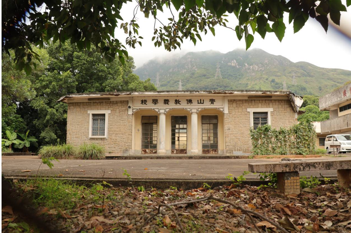
East elevation of the Castle Peak Buddhist School Main Building. Southeast corner of ceiling collapsed.
