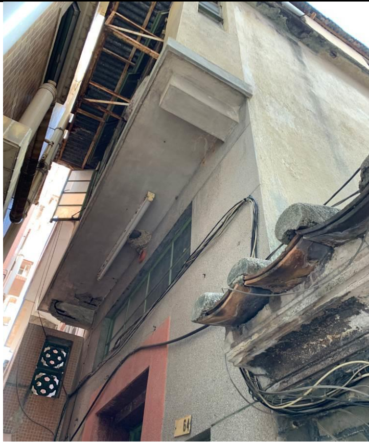
Figure 9. No. 64, Yan Shau Wai (YSW08), a three-storey village house with a flat roof. It has a balcony at the first floor. The front elevation of the ground floor is finished in Shanghai plaster, the side elevations are plastered.
