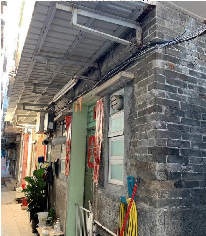
Figure 34. No. 69, Fan Tin Tsuen (FTT15). A traditional Chinese vernacular brick house with a granite base. The building is one-half-one-courtyard in plan. It has plastered relief under eaves on the front façade (blocked by modern addition of door canopy).
