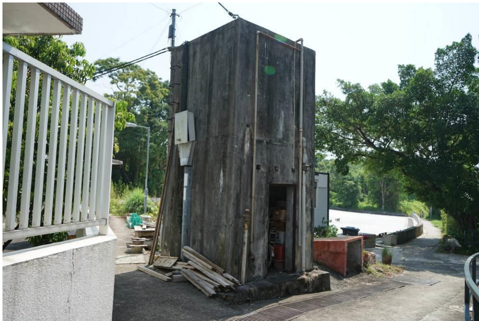
Figure 138. Pump House (PUT12). It is constructed of reinforced concrete. A cat ladder made of metal is attached to the side of the structure. It is currently used as a storage space by the villagers.
