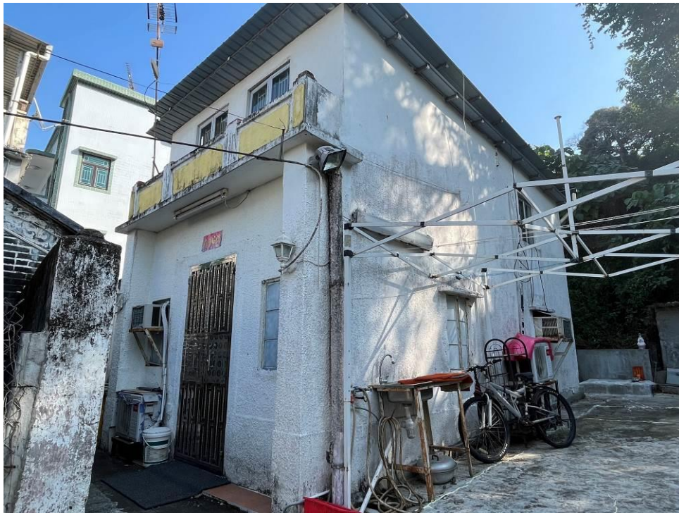
Figure 127. No. 52, Lok Ma Chau Tsuen (LMC15), a two-storey building village house with a flat roof. The entrance is recessed and has a decorative parapet wall above. The exterior is painted in white.
