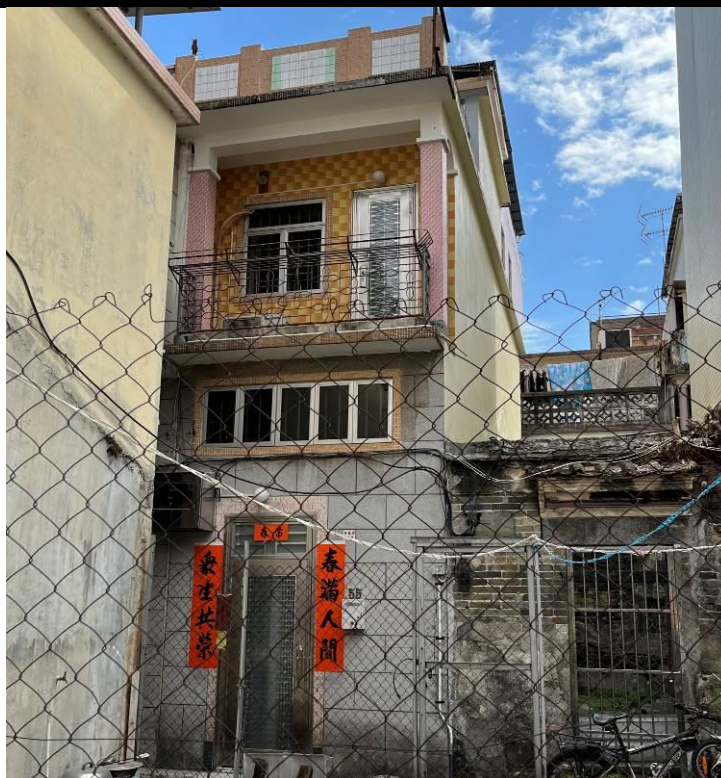
Figure 87. No. 55, On Lung Tsuen (OLT04), a two-storey village house with a flat roof. The building has a high-ceiling ground floor and a balcony with two square corner columns. The front façade of the ground floor is finished in Shanghai plaster and the upper floor is finished in ceramic tiles. The remaining facades is painted in yellow. There is a mosaic-tiled parapet wall on the roof.
