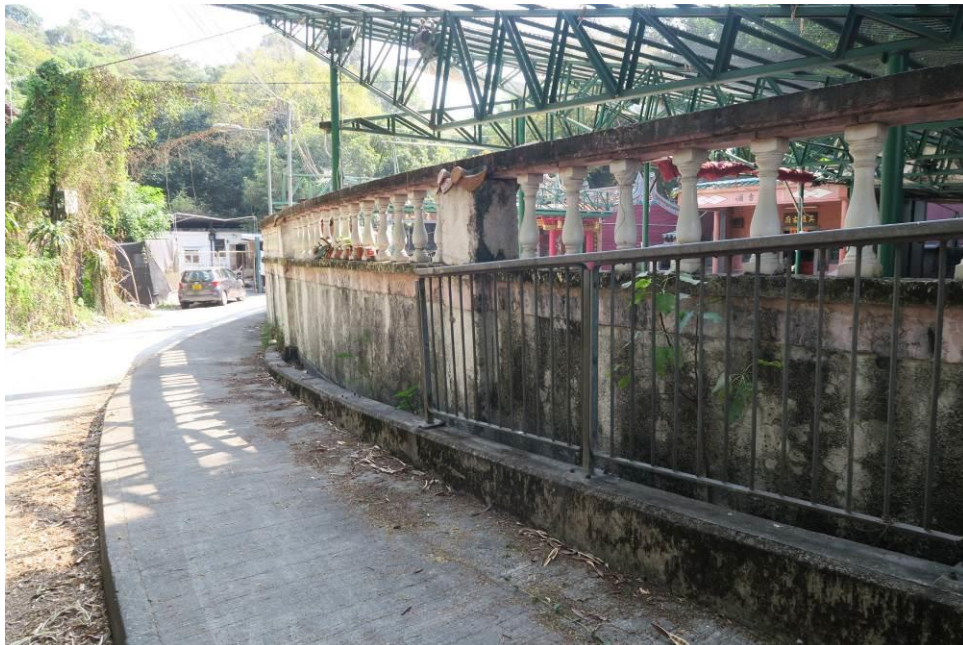
Figure 164. Enclosing wall of Tin Tak Heroes Temple. The site is bounded by an enclosing wall, formed by a concrete wall and a series of vase-shaped balustrades on top.
