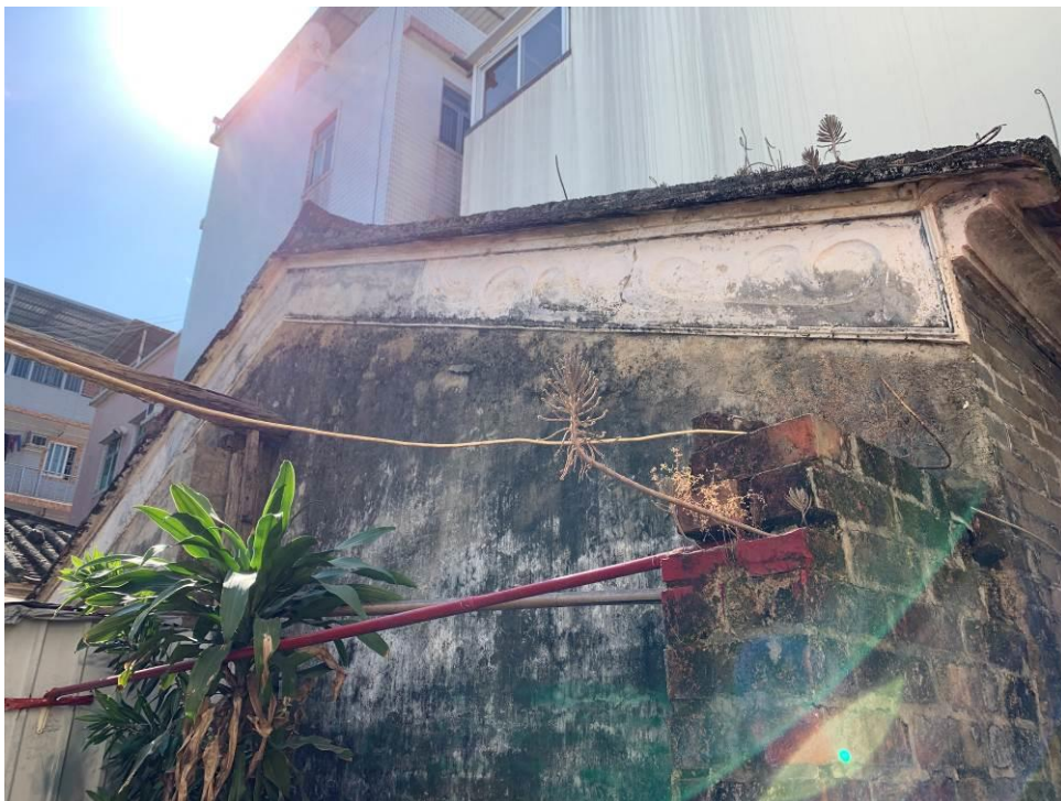
Figure 18. No. 50, Tung Chan Wai (TCW07), a traditional Chinese vernacular single-storey brick building. The building is in a one-hall rectangular plan with its walls supporting the pitched roof. It is decorated by the plastered relief of geometric pattern under eaves on its side elevation.
