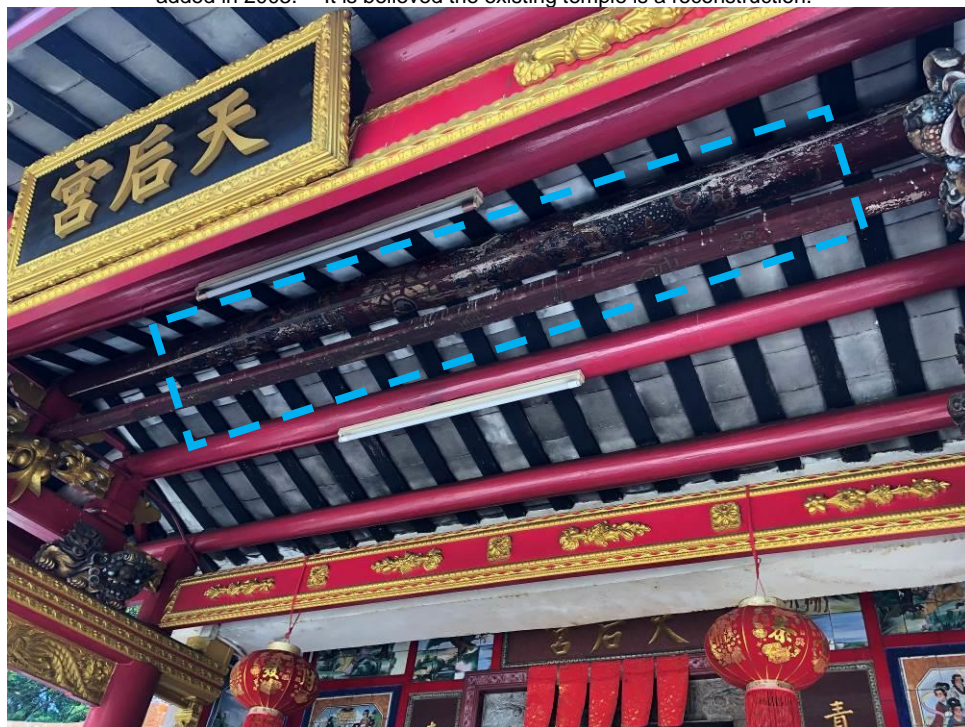
Figure 168. Roof structure of the front porch, Tin Hau Temple. It is observed that the ridge purlin (脊標) and a ridge tiebeam (脊枋) at the front porch of the current Tin Hau Temple (highlighted in blue) are possibly reusing the ridge purlin from an older temple. Decoration with strong Taoism symbols such as the Eight Trigrams (八卦), the Yin-Yang fish (陰陽魚), lotus patterns etc. have been painted elaborately on the ridge purlin, while the ridge tiebeam has four idealized Chinese characters ( “元亨利貞” ) painted on it with one 16-petal chrysanthemum painted in between each character.
