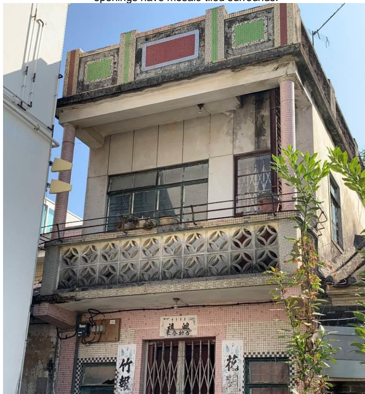
Figure 122. No. 38, Lok Ma Chau Tsuen (LMC10), a two-storey village house. The building has a balcony with two round corner columns and a parapet wall on the flat roof. The front façade of the ground floor and the parapet wall are finished in mosaic tiles, while the first floor is finished in Shanghai plaster.
