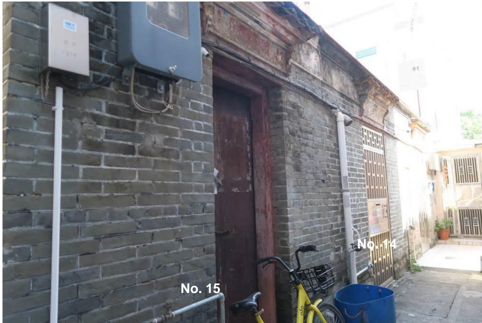
Figure 131. Nos. 12-15, Pun Uk Tsuen (PUT05, PUT06, PUT07 and PUT08). They are a row of Chinese vernacular brick houses. Each in a one-hall-one-courtyard plan.
