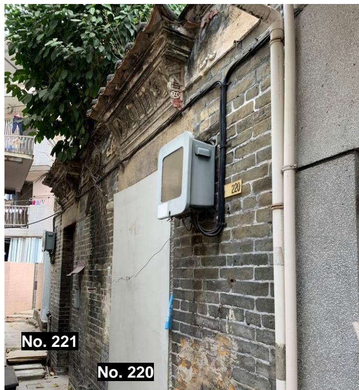
Figure 46. Nos. 220-221, Fan Tin Tsuen (FTT36 and FTT37). They are two residential units in a traditional Chinese vernacular house. Each has a one-hall-one-courtyard plan. Plastered relief can be found under eaves and on door canopy.
