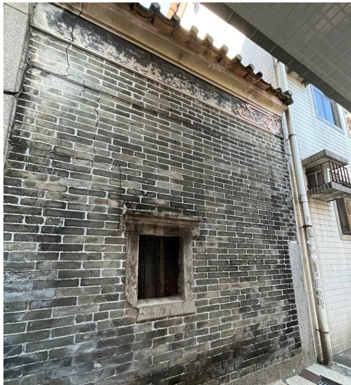
Figure 30. No. 17, Fan Tin Tsuen (FTT07), a traditional Chinese vernacular single-storey house. Plastered relief can be found under eaves. Front elevation is not accessible.
