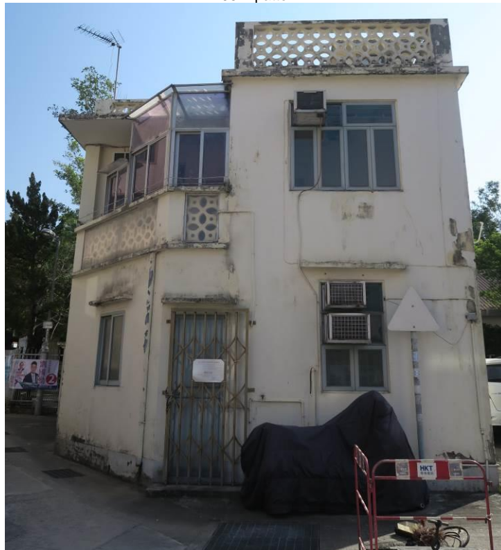
Figure 150. No. 55, Mai Po San Tsuen (MPT09), a two-storey village house with pentagon plan. It has a balcony on the first floor which was possibly enclosed in a later alternation/ addition work. The building is vacant but listed as a government land. It was probably used as the Mai Po Tsuen Recreation Centre with the Former Kwun Ying School at its back before.
