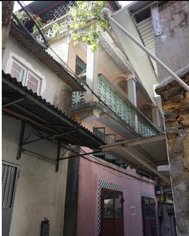
Figure 81. No. 23B, Wing Ping Tsuen (WPT03), a two-storey village house with a flat roof. The building has a high-ceiling ground floor and a balcony on the first floor. Archways are formed between the three columns and the external wall on the balcony. The parapet walls on the balcony and on the roof have geometric pattern elements. The front façade is finished in mosaic tiles.
