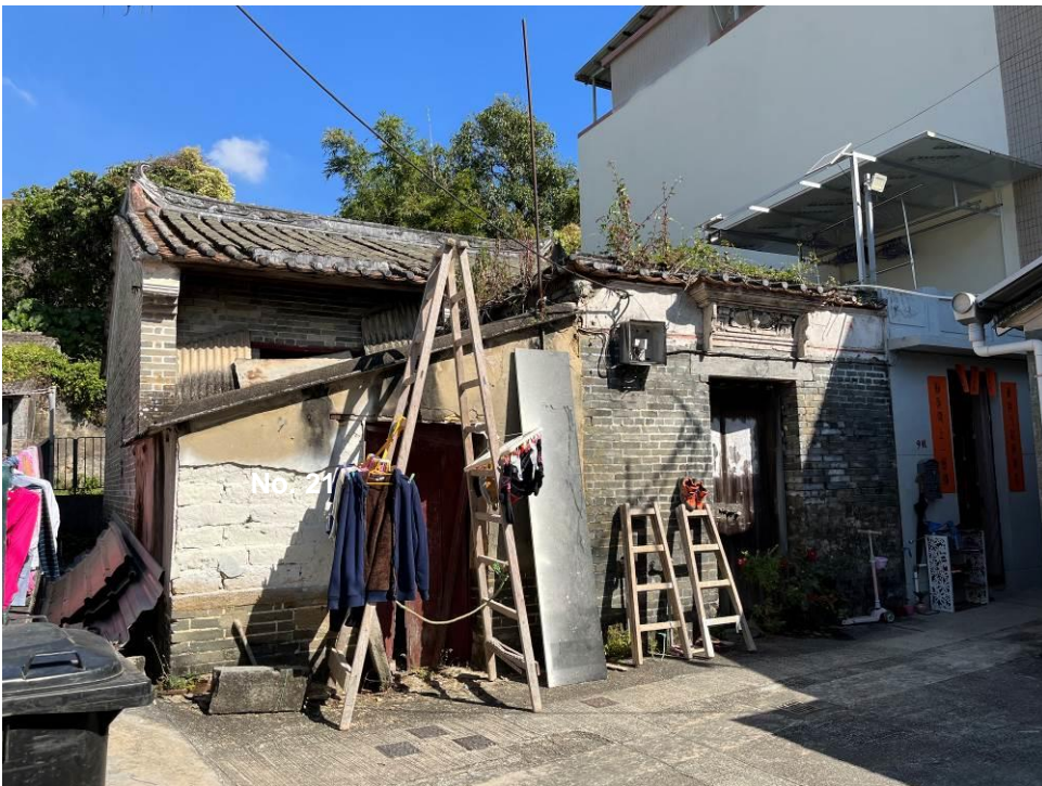
Figure 130. Nos. 10-11, Pun Uk Tsuen (PUT03 and PUT04), a traditional Chinese vernacular brick house with two residential units under the same roof. The building has a pitched roof, the flat main ridge has curled-up ends. No. 11 is in a one-half plan, the original front courtyard is altered with a shed roof. No. 10 is in a one-half-one-courtyard plan. It is decorated by the plastered mouldings of auspicious motifs on door canopy.
