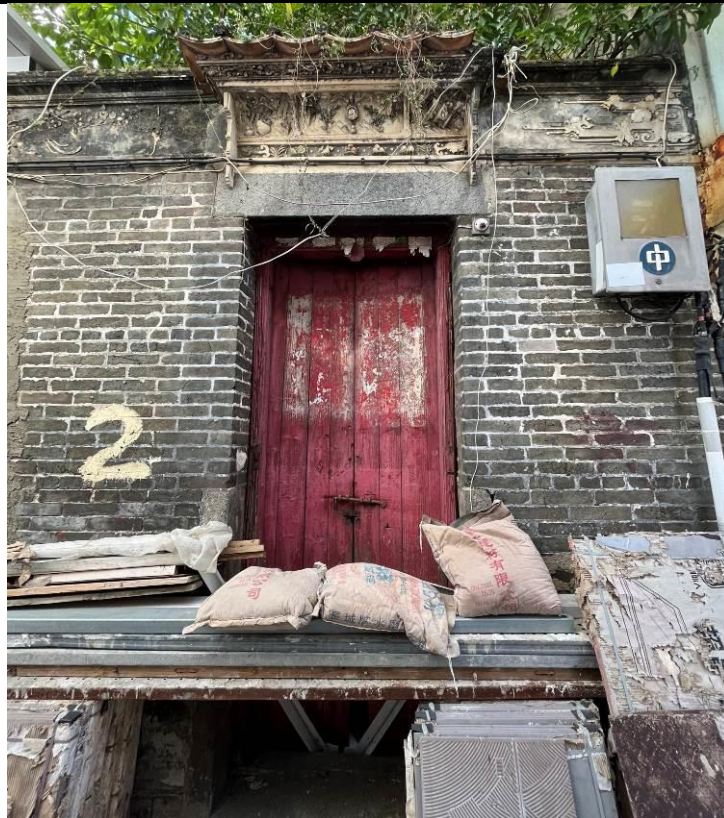
Figure 97. No. 2, San Lung Tsuen (SLT01). It is traditional Chinese vernacular single-storey brick building. It is in a one-hall-one-courtyard plan. The building is decorated by the plastered relief of auspicious motif on the door canopy as well as plastered relief of flora and ruilong (夔龍) patterns on wall frieze.
