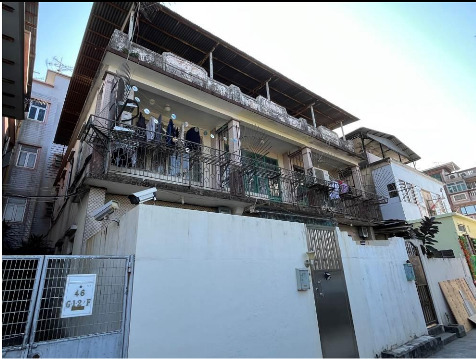
Figure 149. Nos. 47-49, Mai Po San Tsuen (MPT08), a two-storey village house with three residential units. The building has a balcony with square columns defining each unit. The parapet wall at the top has plastered mouldings of flora motifs and "1967" pattern.
