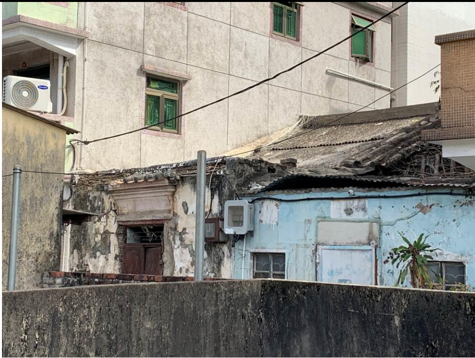
Figure 5. No. 84B, Yan Shau Wai (YSW10), a traditional Chinese vernacular pitched-roof building. It is in a one-half-one-courtyard plan. The entrance has a decorative door canopy and a window grill of geometric pattern above the metal door.
