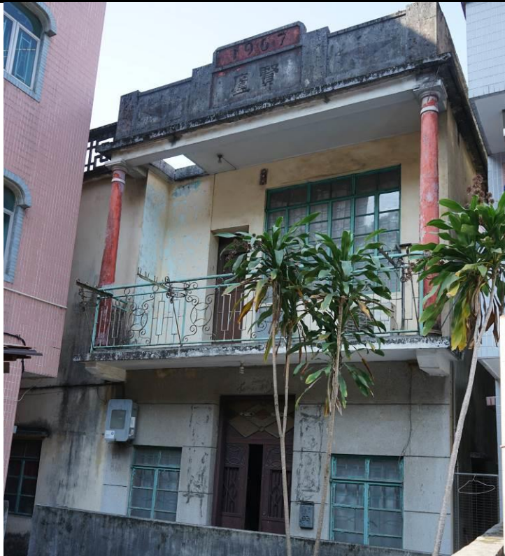
Figure 147. No. 12, Mai Po San Tsuen (MPT06), a two-storey village house in a L-shape plan. The building has a balcony with two round corner columns. The parapet wall on the roof has plastered mouldings of “1967” and Chinese characters of “賢廬”. The front façade of the ground floor is finished in Shanghai plaster and the other facades are painted in pale yellow.
