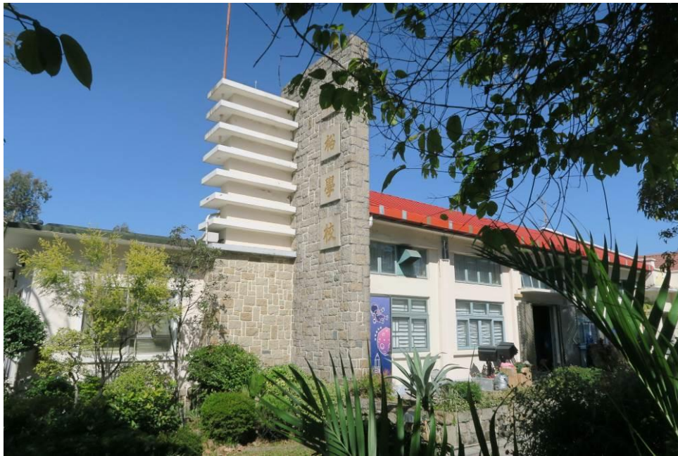
Figure 11. Lightning Rod on a L-shaped granite wall. For the wall backing the south annex, the upper part is constructed of concrete with horizontal strips projecting out from the surfaces, while the lower part remains to be granite blocks. The other wall is constructed of granite blocks. Plates with the Chinese characters of the school (“惇裕學校”) are hung on this wall.
