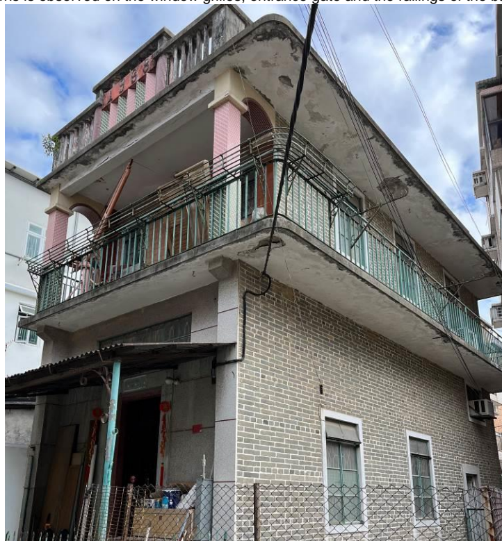
Figure 74. No. 239A1, Fan Tin Tsuen (FTT45), a two-storey village house with a high-ceiling ground floor and a flat roof. The building has a balcony extending across the front and the side of the building. The balcony has two archways at both sides, formed between the mosaic-tiled square columns and the external wall.
