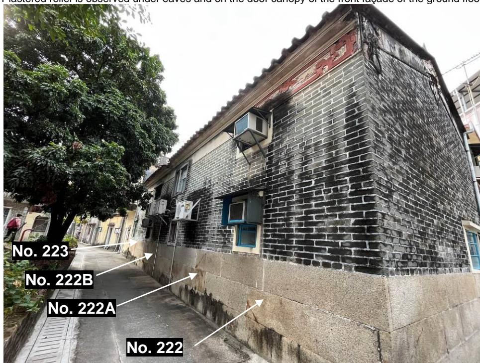
Figure 52. Nos. 222, 222A, 222B and 223 (FTT38, FTT39, FTT40 and FTT41), Fan Tin Tsuen, back elevation.
