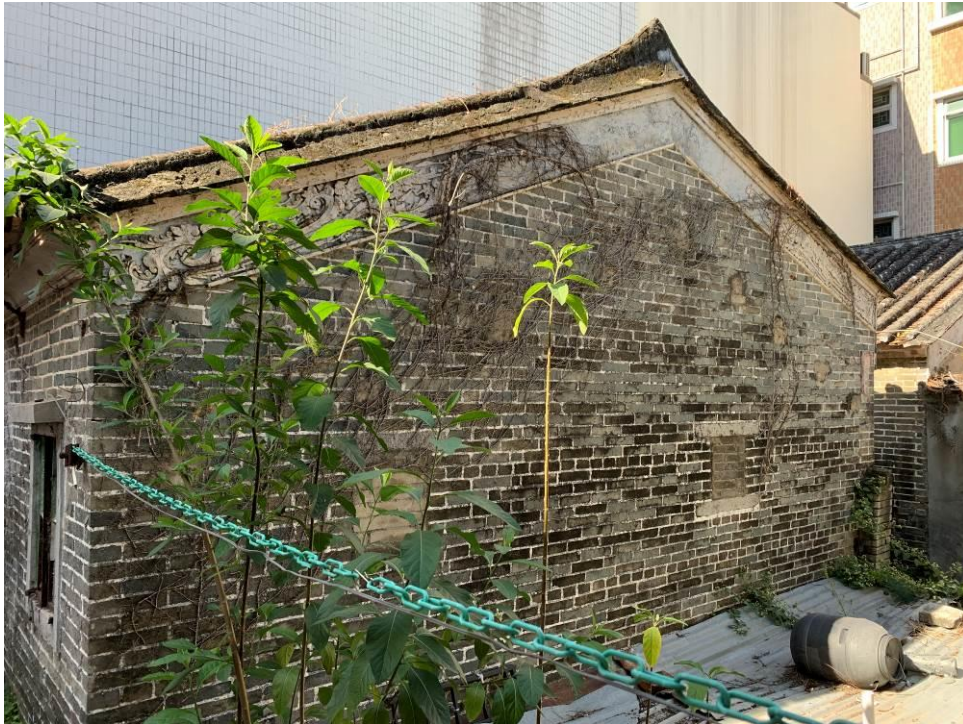
Figure 17. No. 43A, Tung Chan Wai (TCW06). The building is in a one-hall rectangular plan with its walls supporting the pitched roof.
