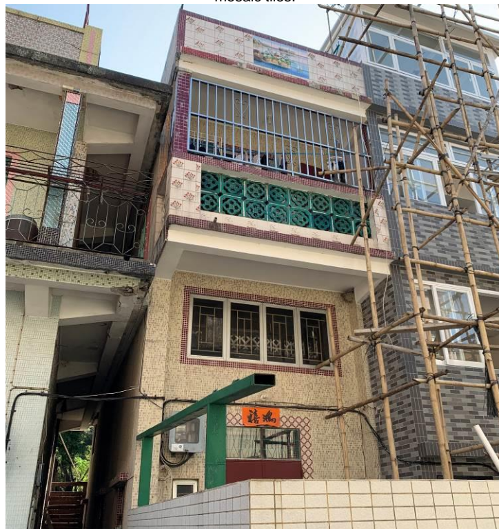
Figure 152. No. 96A, Mai Po San Tsuen (MPT13), a two-storey village house with a flat roof. The building has a high-ceiling ground floor and a balcony with two square corner columns. The parapet wall on the roof has scenery painted on the ceramic tiles. According to the village elders, this is a culture of people originated from Fujian (鶴佬). The front façade is finished in ceramic tiles.
