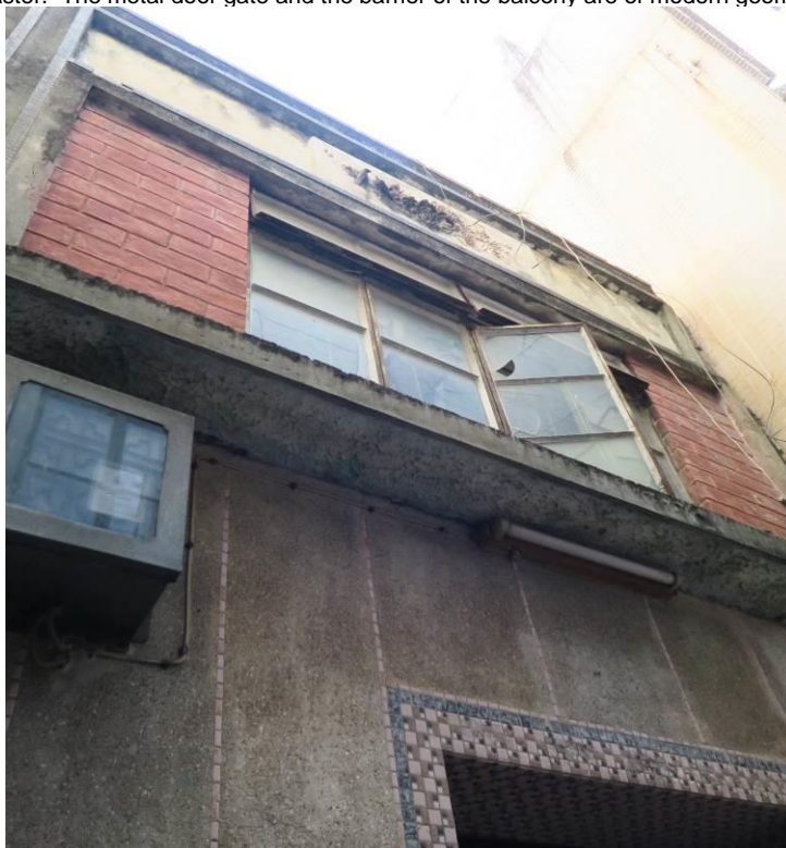
Figure 58. No. 37, Fan Tin Tsuen (FTT14), a two-storey house with a flat roof. The ground floor is finished with Shanghai plaster and mosaic tiles around the entrance, the first floor is finished with red bricks. The parapet wall on the roof is decorated with plastered relief with flora motif.
