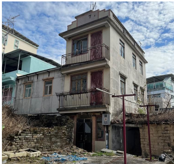
Figure 8. No.51, Yan Shau Wai (YSW07), a three-storey village house with a flat roof. It has a balcony at the first and second floor. The front elevation is finished in ceramic tiles while the side elevations are plastered. The parapet wall on the roof indicates the building was probably constructed in the 1970s.
