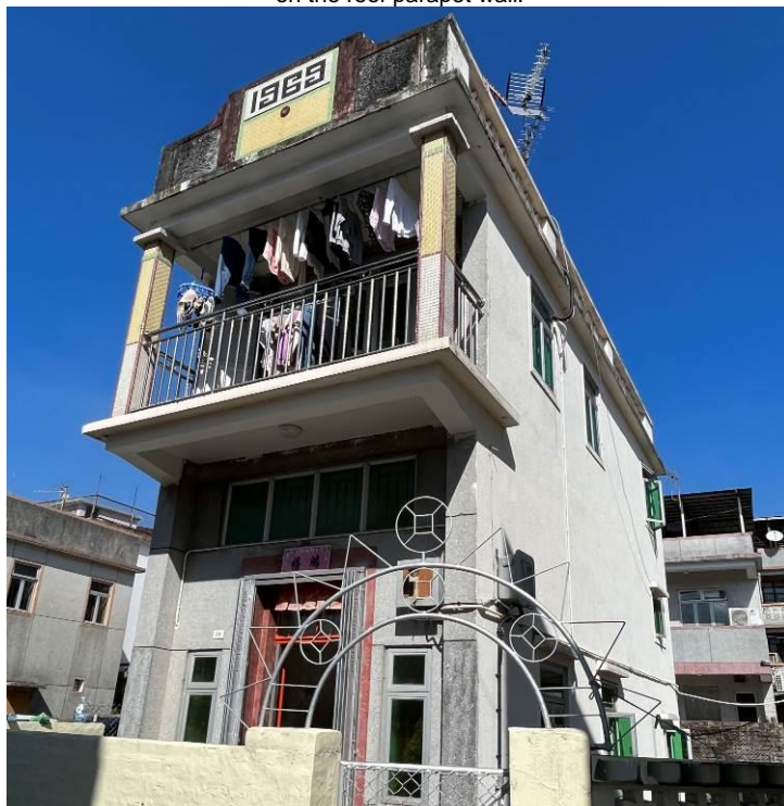
Figure 136. No. 50, Pun Uk Tsuen (PUT11). The building is a two-storey village house with a flat roof. It has a high-ceiling ground floor and a balcony with two square corner columns decorated with mosaic tiles. Pattern of "1969" is observed on the roof parapet wall. The front façade of the building is finished in Shanghai plaster.
