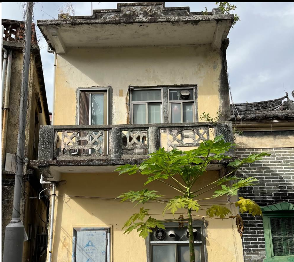
Figure 71. No. 224, Fan Tin Tsuen (FTT42), a two-storey village house with a flat roof and a balcony on the first floor. The exterior is painted in yellow. The balustrade of the balcony is probably constructed of concrete with geometric patterns.
