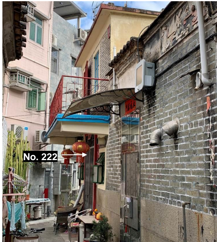
Figure 49. No. 222, Fan Tin Tsuen (FTT38), front elevation. The building has a balcony which extends across the front and the side of the building.
