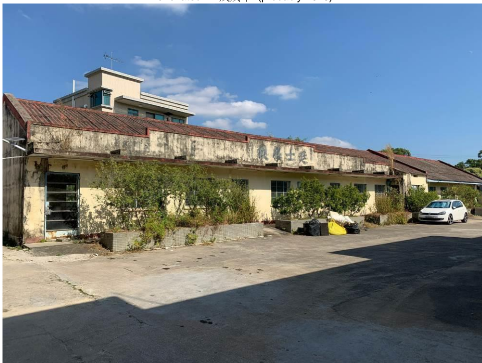
Figure 108. Ting Sze School (CTT08). It was registered on 25 th March, 1946 22 . It is a typical single-storey village school structure with a pitched roof. The front elevation has a parapet wall. It is in Utilitarian style. The school has two classrooms with an extension to its southeast end. The external wall is painted in light yellow.
