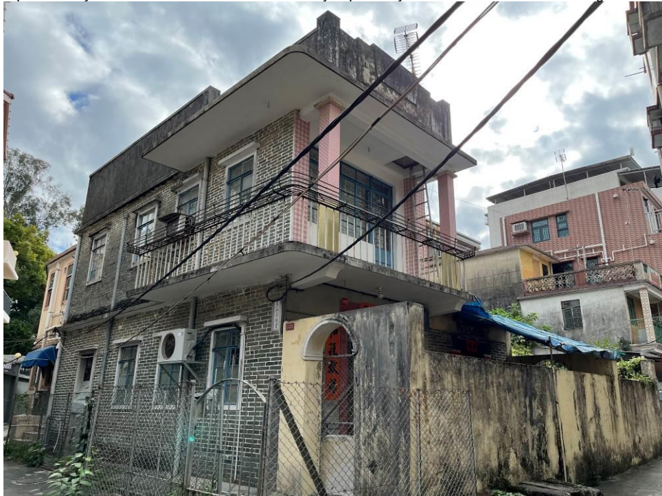
Figure 72. No. 225, Fan Tin Tsuen (FTT43), a two-storey village house with a flat roof. It has a balcony extended across the front and the side of the building. The balcony has two square corner columns which are finished in mosaic tiles. The front elevation of the ground floor is finished with Shanghai plaster, the first floor is painted in white.
