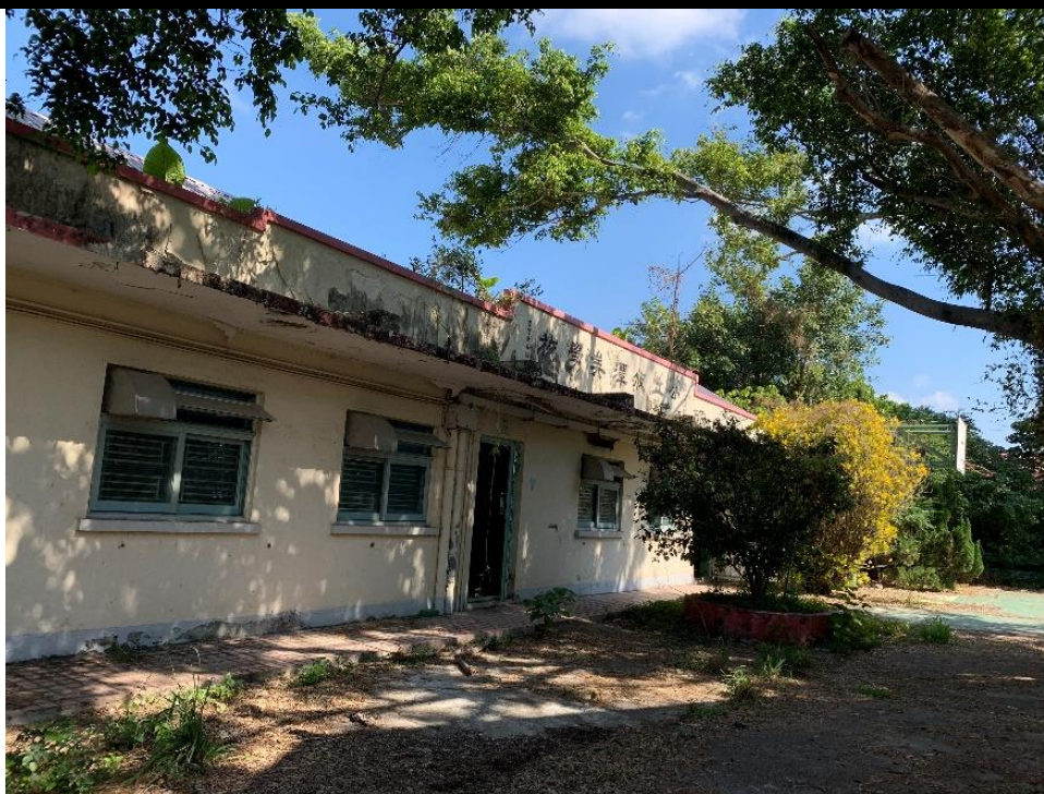
Figure 175. Yau Tam Mei Public School. The school was established in 1931 as a private school by Chu Shau Ki (朱壽棋), namely Tak San School (德新學校). The school was re-established as Yau Tam Mei School (攸潭美學校) in 1939 44 . In 1946, the school has been government-subsidized since. The name of the school was changed to Yau Tam Mei Public School (攸潭美公立學校) to indicate its subsidiary by the government.
