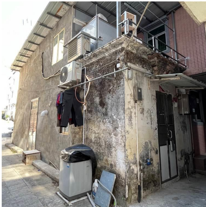
Figure 104. No. 56, Chau Tau Tsuen (CTT05), two-storey village house with a shed roof. The building was probably undergone reconstruction that the original front courtyard was retained while the back hall has been rebuilt. Plastered reliefs can be found on the door canopy on the front elevation.
