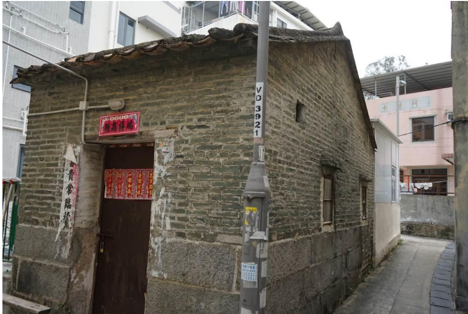
Figure 39. No. 85G, Fan Tin Tsuen (FTT20), a traditional Chinese vernacular single-storey house. The building is constructed of grey bricks with its walls supporting the pitched roof. The lower courses of the brick walls are constructed of granite blocks. The window openings on the side wall are metal framed with projected window label mouldings above.
