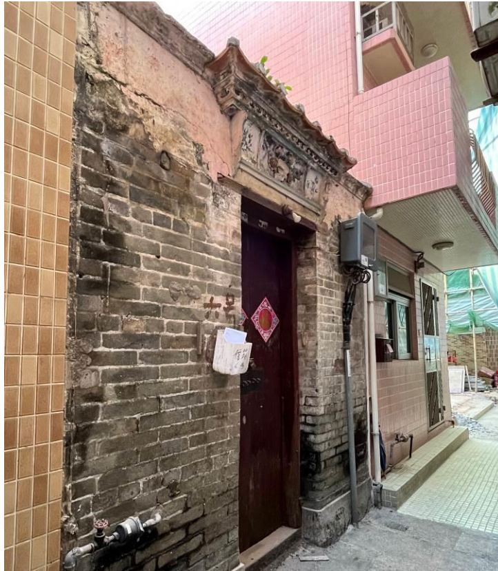
Figure 111. Structure Between No. 5 and No. 7, Shek Wu Wai (SWW01). It is a traditional Chinese vernacular single-storey brick building in a one-hall-one-courtyard plan.
