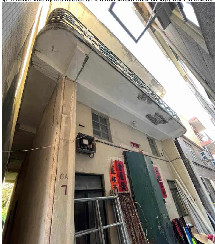
Figure 134. No. 6A-7, Pun Uk Tsuen (PUT02). It is a two-storey village house with a high-ceiling ground floor. It has a balcony extending across the front elevation and side elevations of the building. The building condition is fair with spalling concrete observed at the bottom of the balcony and the projected roof slab.
