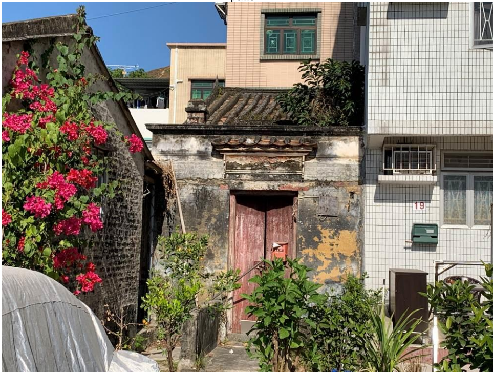
Figure 102. No. 18, Chau Tau Tsuen (CTT03), a single-storey brick house in a one-hall-one-courtyard plan. The building has a pitched roof. The building is decorated with plastered relief on the door canopy, but it is deteriorating.
