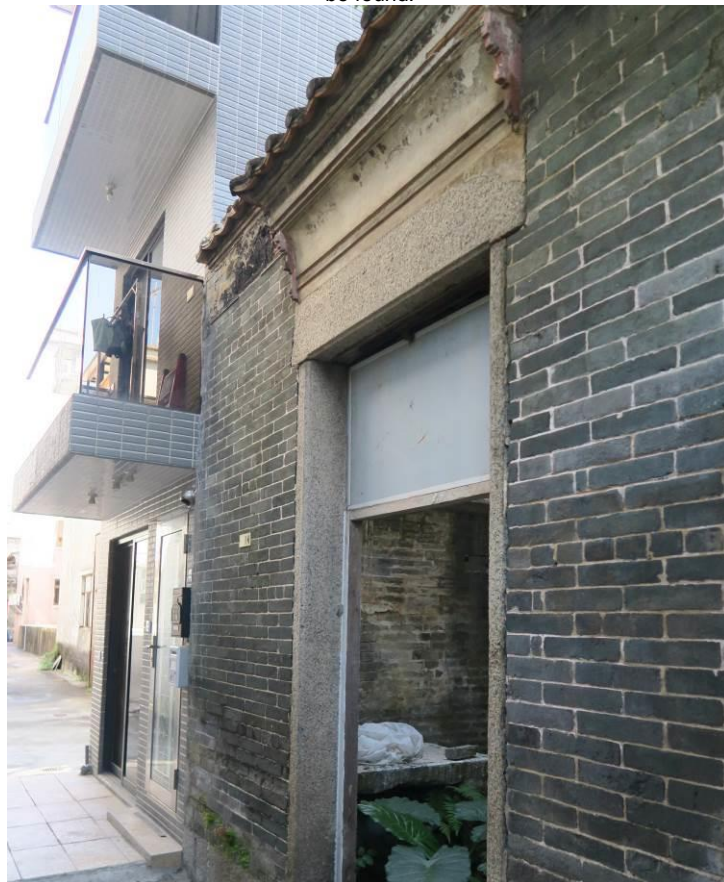
Figure 28. No. 14, Fan Tin Tsuen (FTT05), a traditional Chinese vernacular single-storey house. Murals and plastered relief can be found but are fading due to lack of maintenance.
