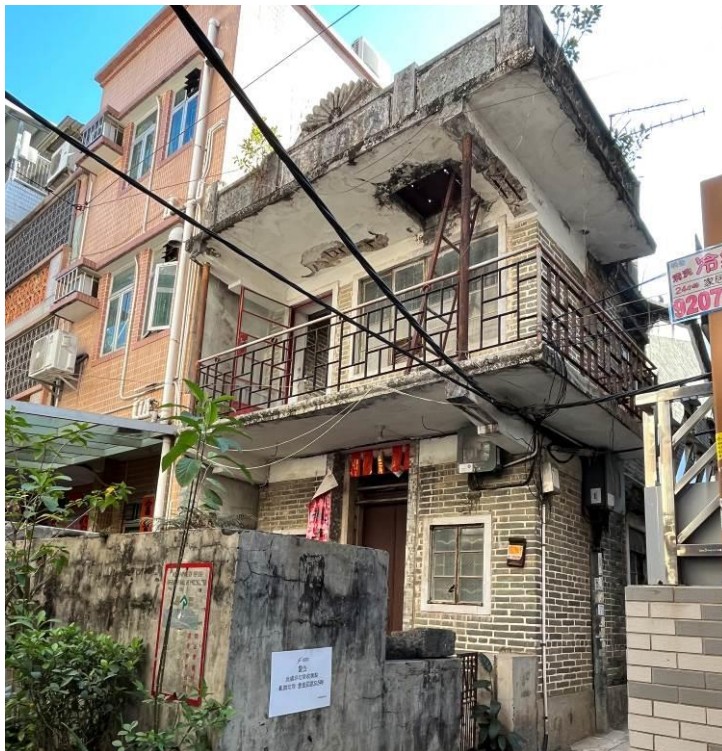
Figure 76. STL657 in Fan Tin Tsuen (FTT49), a two-storey flat-roof village house. The building has a balcony extending across the front and the side of the building. The parapet wall on the roof has “1962” inscribed and a plaster sculpture of semi-flower form.
