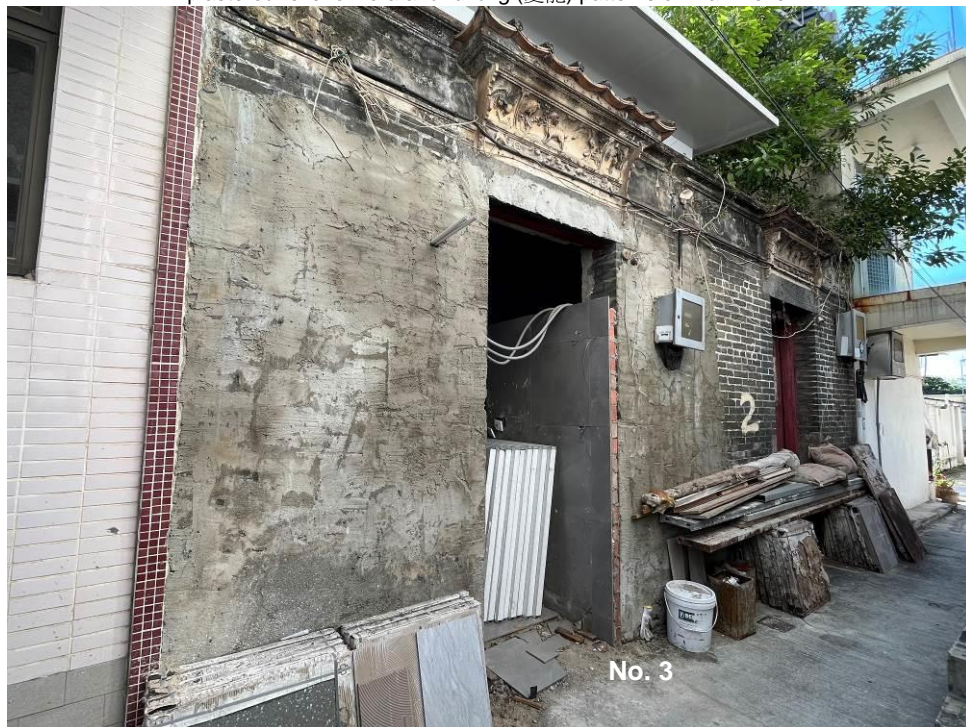
Figure 98. No. 3, San Lung Tsuen (SLT02), a traditional Chinese vernacular single-storey brick building. It is in a one-hall-one-courtyard plan. It is decorated by the plastered relief of flora motif on the door canopy. The building is undergoing renovation.
