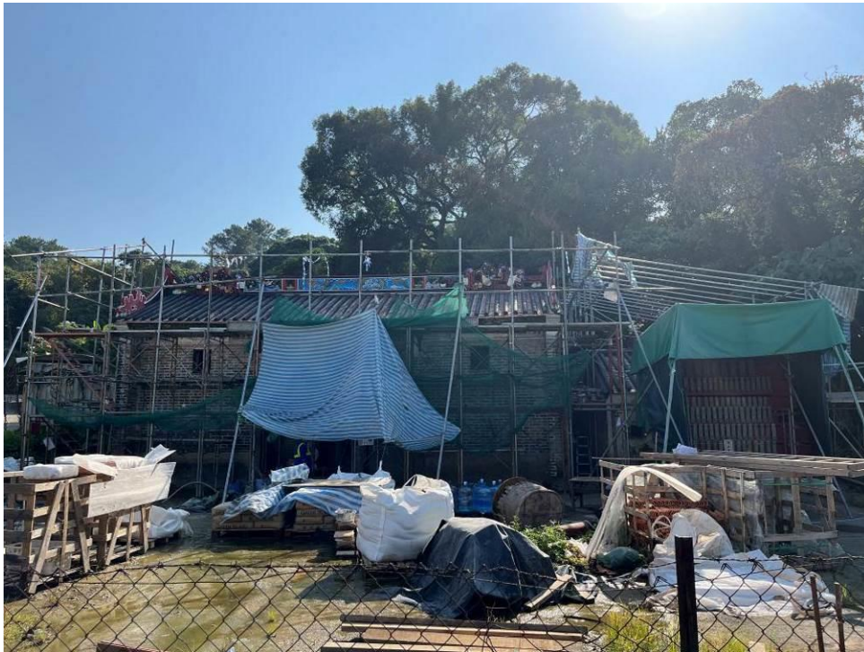
Figure 47. Front elevation of Mi Tak Study Hall showing the Main Block and the Ancillary Building (behind the altar).
