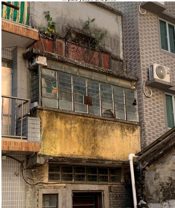
Figure 20. No. 15, Tung Chan Wai (TCW05), a three-storey village house with a flat roof. The building has an enclosed balcony on its first floor with a parapet wall on top. It is speculated the second floor of the building is a late addition.
