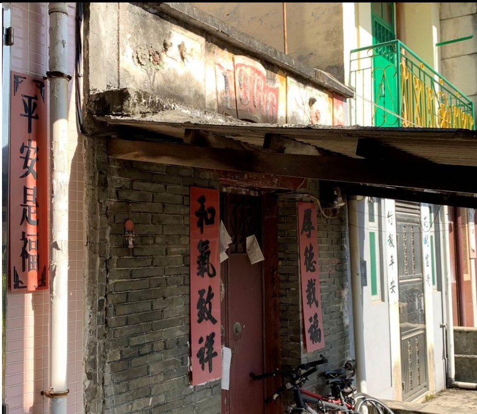
Figure 101. No. 3, Chau Tau Tsuen (CTT01), a single-storey brick house in a one-hall-one-courtyard plan. The building has a pitched roof. The parapet wall has plastered relief of flower and bird motifs and plastered mouldings of a scroll and “1966” pattern.
