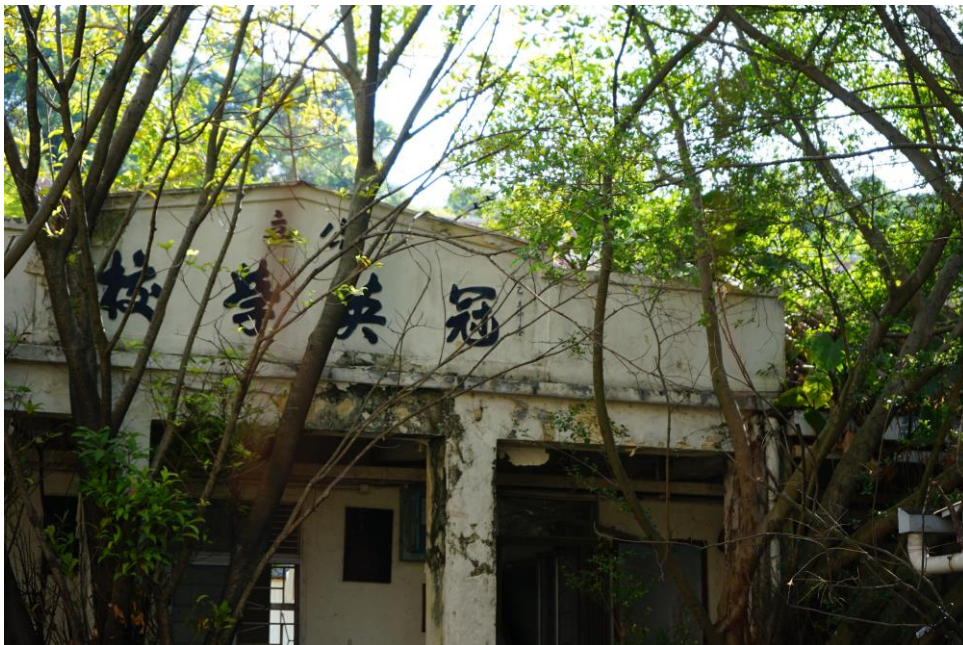
Figure 160. Former Koon Ying Public School (MPT20). The main building has a stepped parapet wall on the roof. It has plastered mouldings of Chinese characters of Koon Ying Public School (“公立 冠英學校”) and 1955 Spring (“乙未仲春”), indicating the establishment year of the school.
