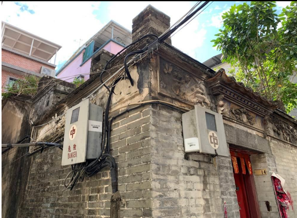
Figure 1. No. 14, Yan Shau Wai (YSW01), a traditional Chinese vernacular pitched-roof building. It is in a one-half-one-courtyard plan. The building is decorated by the plastered mouldings of flora and treasure motifs on the wall frieze on the front and side elevations, as well as on the door canopy.
