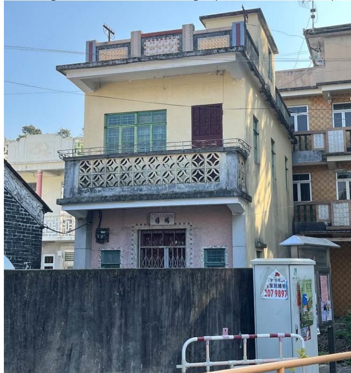
Figure 120. No. 34, Lok Ma Chau Tsuen (LMC08). It is a two-storey village house with a flat roof. The barrier of the balcony at the first floor is formed by the traditional Chinese coin patterns. The parapet wall on the roof and the front façade of the ground floor are finished in mosaic tiles. The remaining facades are painted in pale yellow.
