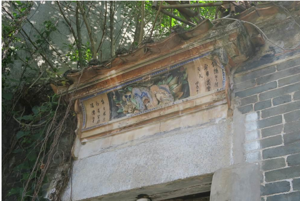
Figure 27. No. 12, Fan Tin Tsuen (FTT04). Decorations including mural on door canopy and plastered relief under eaves can be found.
