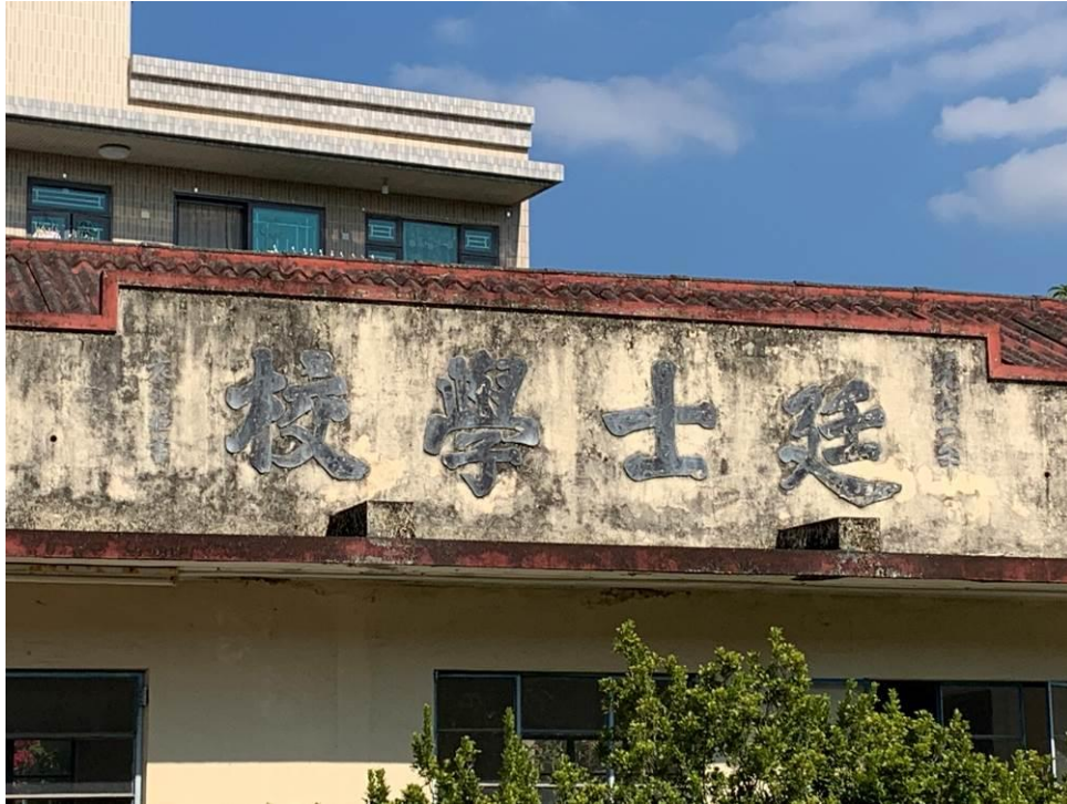
Figure 109. Ting Sze School (CTT08). According to the plastered mouldings on the parapet wall, the existing school building was erected in 1961.
