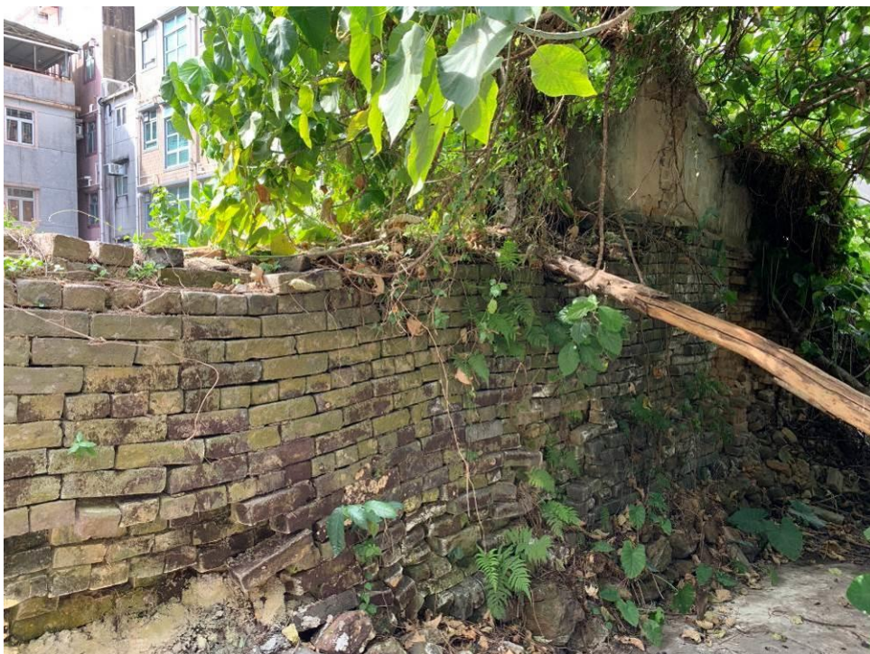
Figure 72. The Northeast Enclosing Wall, layered in a “三順一丁” manner, has deformed and covered in heavy vegetation.
