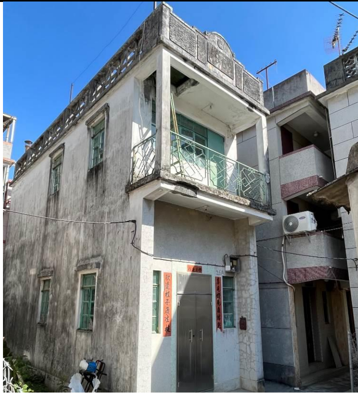
Figure 135. No. 29, Pun Uk Tsuen (PUT10). The building is a two-storey village house. It has a high-ceiling ground floor and a balcony with two square corner columns. The balcony is connected to the flat roof by a ladder. Pattern of "1969" is observed on the roof parapet wall.
