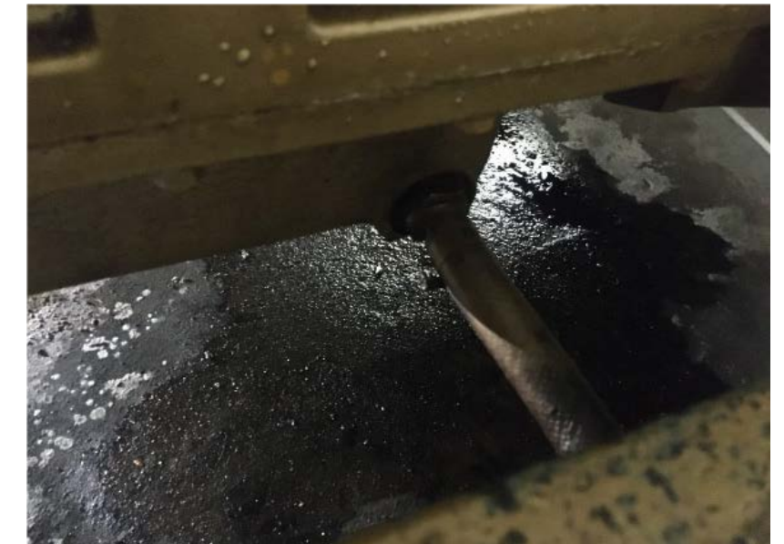
| Signs of land contamination – leakage from diesel storage and backup generator
