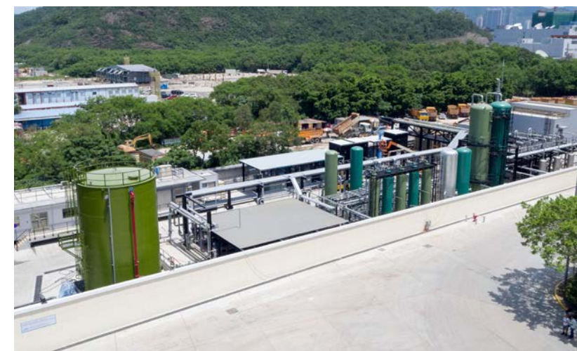
| SENT Landfill – Landfill Gas Utilisation Facility
