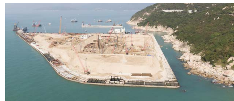
| Site formation and pilling works at the artificial island in progress at I-PARK1 (December 2021)
