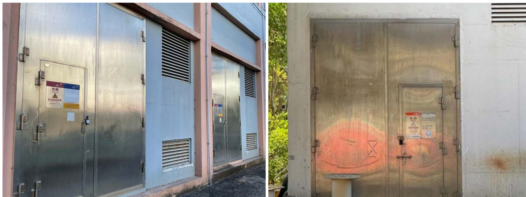
| Potential land contamination hot spot – place for housing transformer
