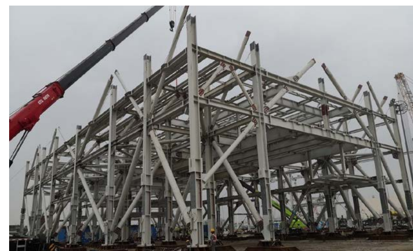
| Steel structure erection for prefabricated electrical and mechanical units at I-PARK1's Prefabrication Yard in Zhuhai (December 2021)
