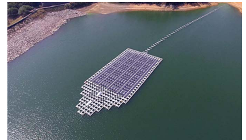
Net-zero Electricity Generation – Floating Solar Generation System at Plover Cove Reservoir
