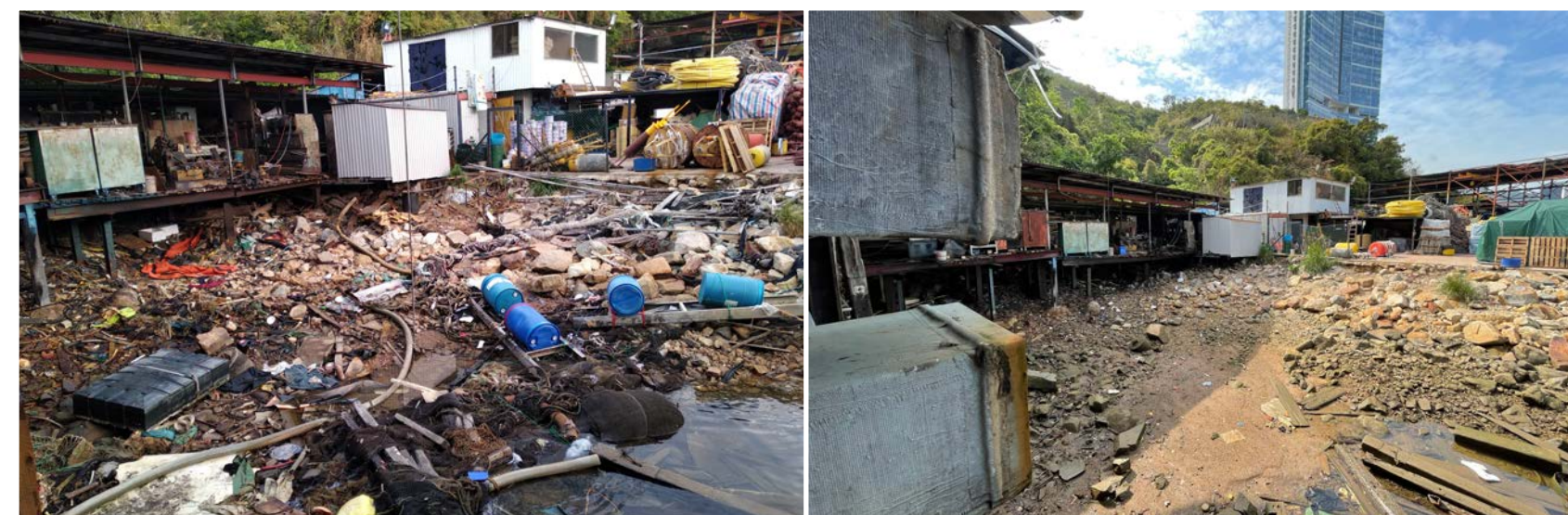
Specialised shoreline refuse clean-up at the Government vacant land between shipyards at Aberdeen Typhoon Shelter (left: before; and right: after clean-up operation)
