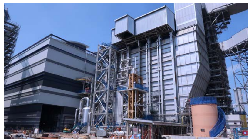
The Hong Kong Electric Company Limited (HEC)'s New Combined Cycle Gas Turbine at Lamma Power Station
