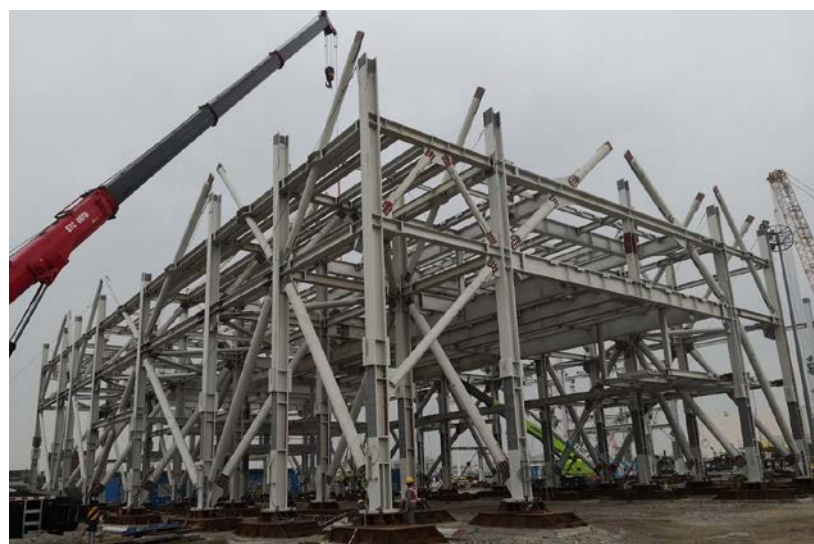
Steel structure erection for prefabricated electrical and mechanical units at I-PARK1's Prefabrication Yard in Zhuhai (December 2021)
