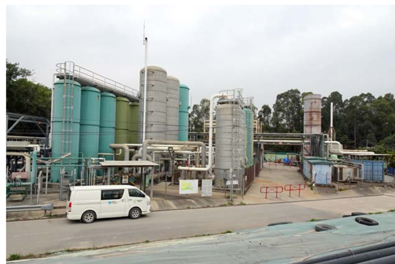
| Landfill Gas Treatment Facility at the NENT Landfill
