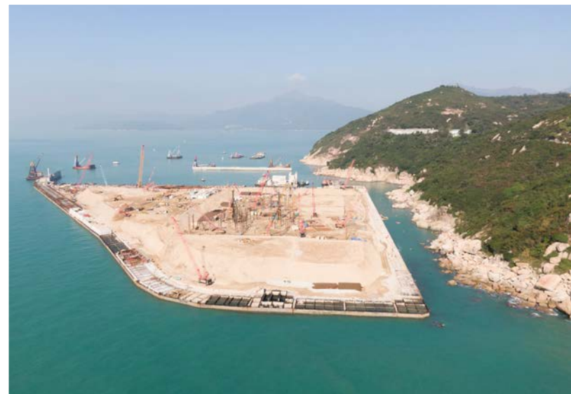
Site formation and piling works at the artificial island in progress at I-PARK1 (December 2021)
