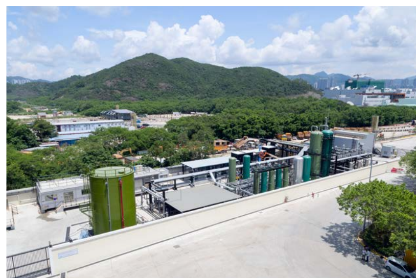
| Landfill Gas Utilisation Plant at the SENT Landfill
