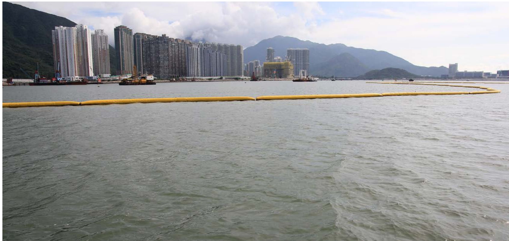
Silt curtain to mitigate water quality impacts
