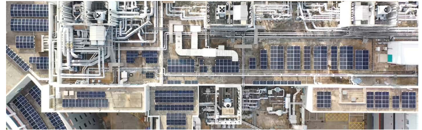
Aerial shot of solar panels installed at the rooftop of the Hong Kong University of Science and Technology (HKUST). The HKUST announced in 2020 that the school would install up to 8 000 solar panels at over 50 campus locations
