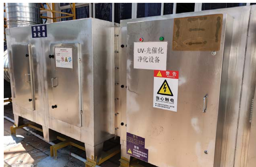
Installation of composite exhaust air treatment system using a combination of UV photocatalytic oxidation and activated carbon adsorption to reduce VOC emissions
