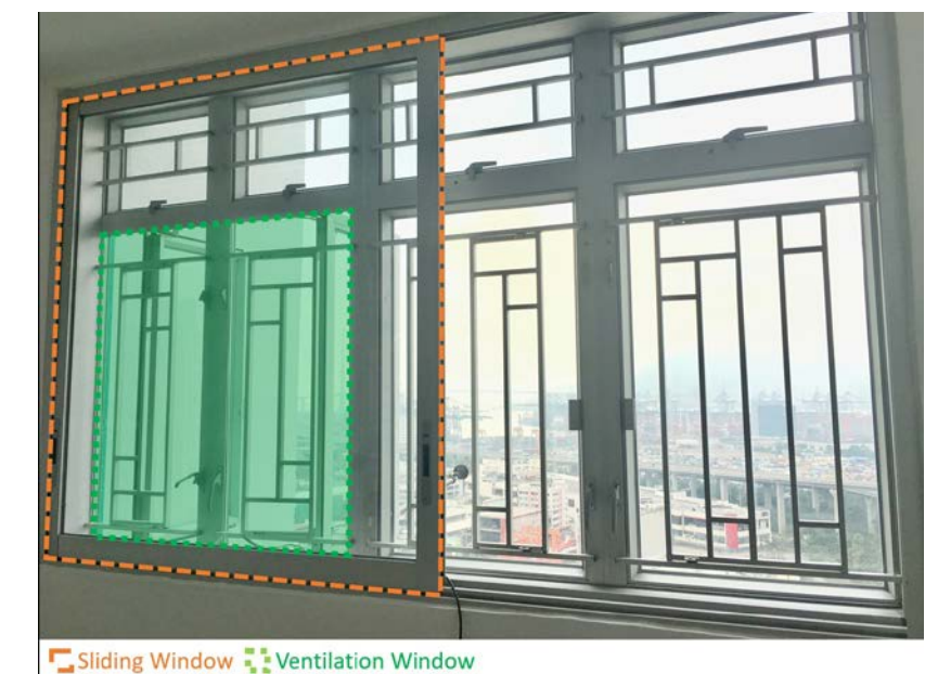
| Baffle type acoustic window at Hoi Ying Estate to mitigate traffic noise from West Kowloon Highway
