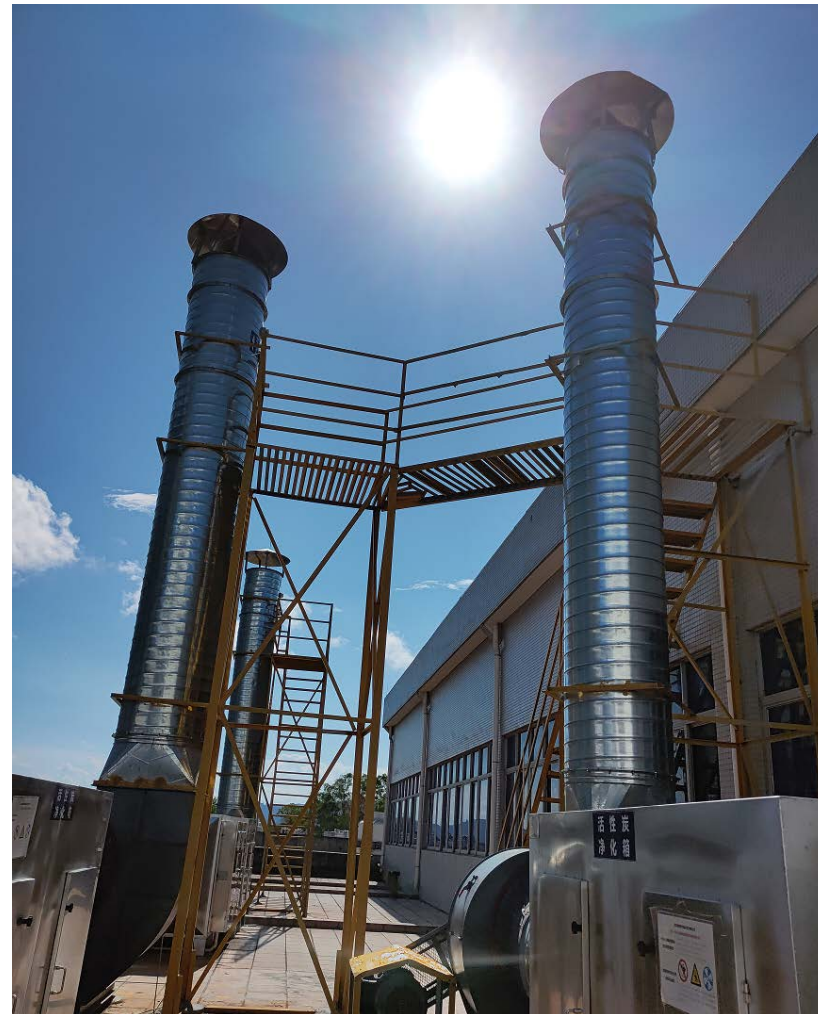
Installation of composite exhaust air treatment system using a combination of UV photocatalytic oxidation and activated carbon adsorption to reduce VOC emissions
