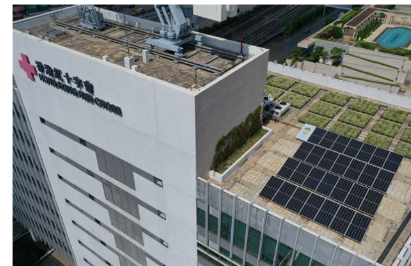
Solar energy generation system installed at Hong Kong Red Cross Headquarters under Solar Harvest
