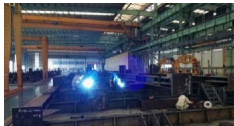
Welding and erection of a steel frame for prefabricated electrical and mechanical units at I-PARK's Prefabrication Yard in Zhuhai (December 2020)
