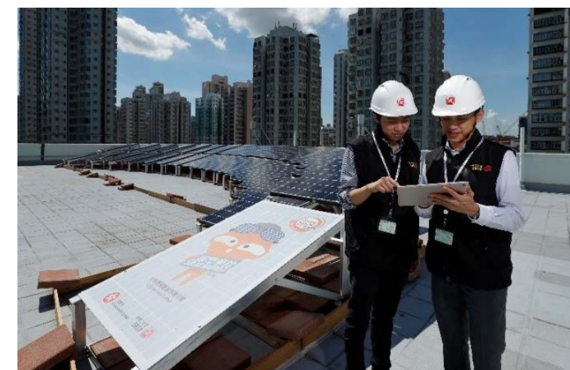
Engineers carried out testing of the solar energy generation system installed under Solar Harvest
