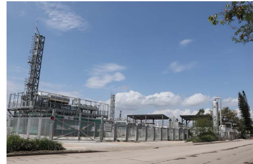
| WENT Landfill Gas Power Generation Project
