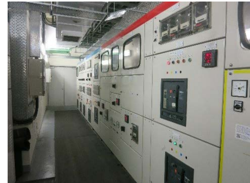
Electrical Installations are covered by the Buildings Energy Efficiency Ordinance
