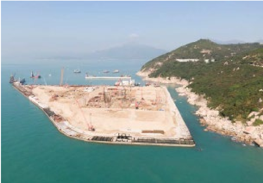
On-site foundation works and steel structure erection for Process Building at the artificial island in progress at I-PARK1 (2022)
