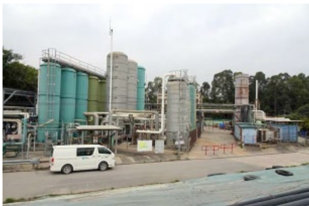
Landfill Gas Utilisation Plant at the NENT Landfill
