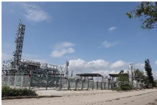
Gas Power Generation Project at the WENT Landfill
