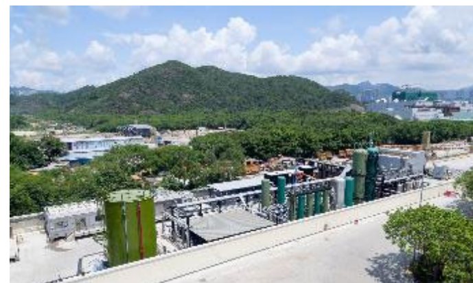
Landfill Gas Utilisation Plant at the SENT Landfill
