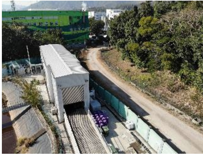
Food Waste Pre-treatment Facilities for food waste / sewage sludge anaerobic co-digestion trial scheme at TPSTW
