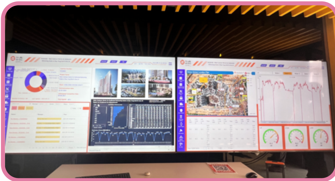
A centralised management platform provides an overview of construction noise monitoring
