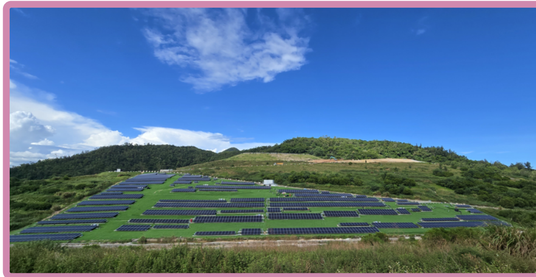
One mega-watt pilot solar farm at SENT Landfill
