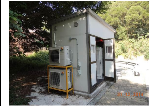
Rectifier of the Charging Facility
