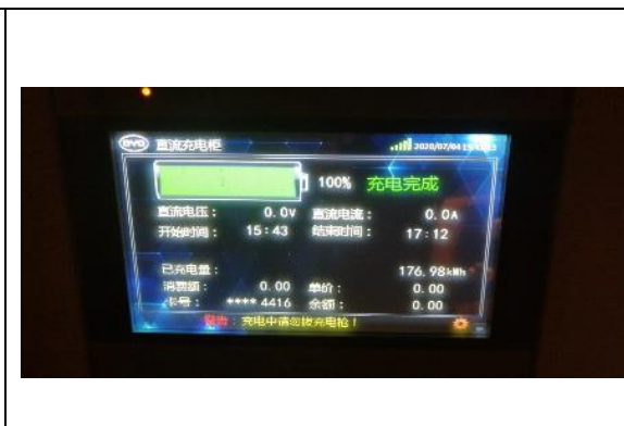
Charging Display Panel for EV
