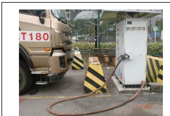
Charging Facility for EV
