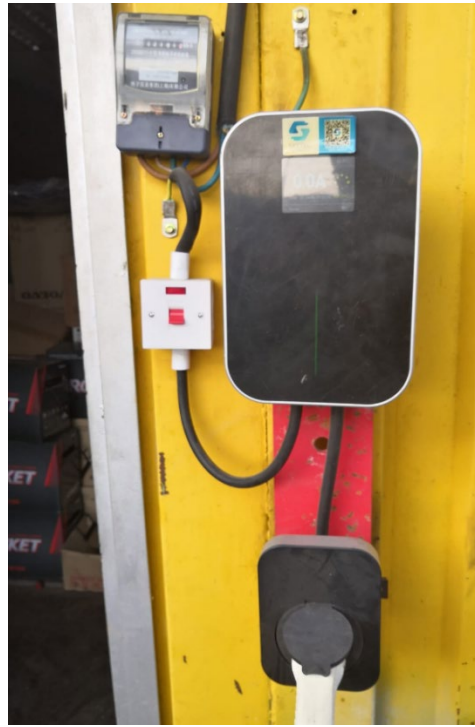
The single-phase 7 kW charger with the electricity meter
