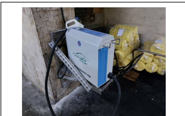
30kW DC charging facility
