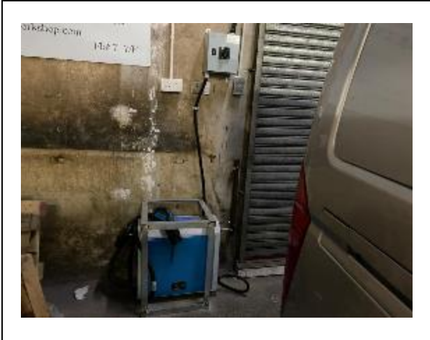
30kW DC charging facility
