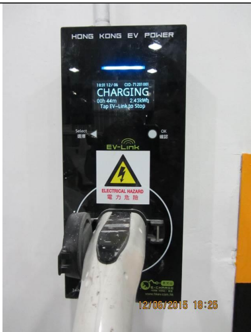
EV Charging Station
