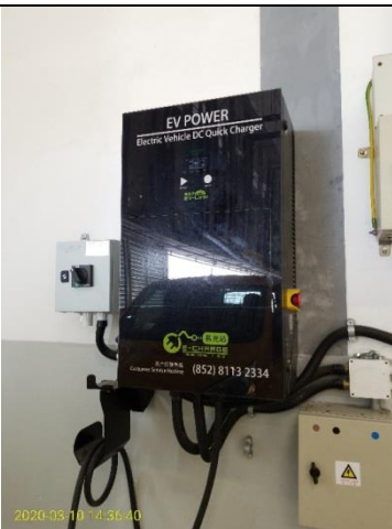
EV Charging Station
