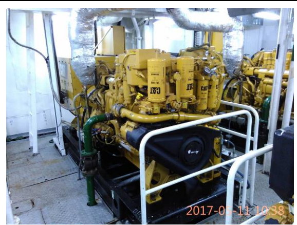
#2 main diesel generator (for propulsion)
