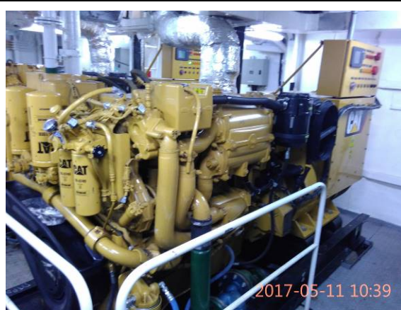
#1 main diesel generator (for propulsion)
