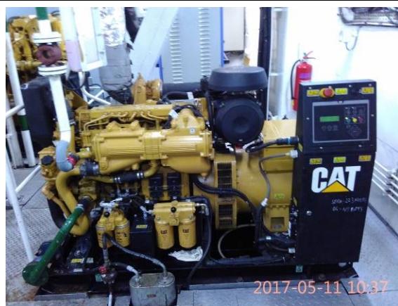
Auxiliary diesel generator
