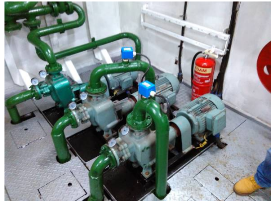
Seawater pumps for seawater scrubbers
