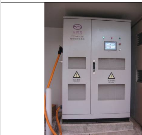
Charging station with charging cable – external view
