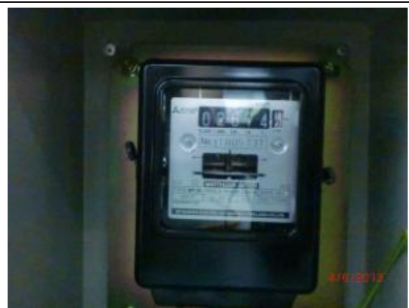
Watt-hour meter at charging station
