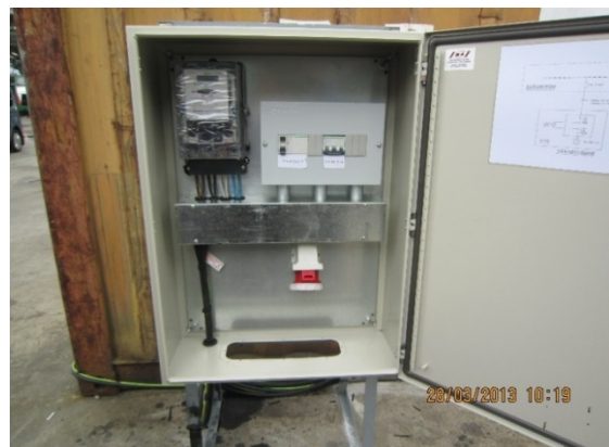
EV-2 – Charging station at TSW depot
