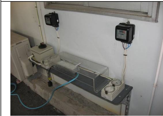
Charging station for the EVs
