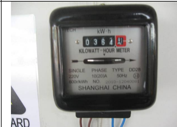
Watt-hour meter of EV-2's charging facility
