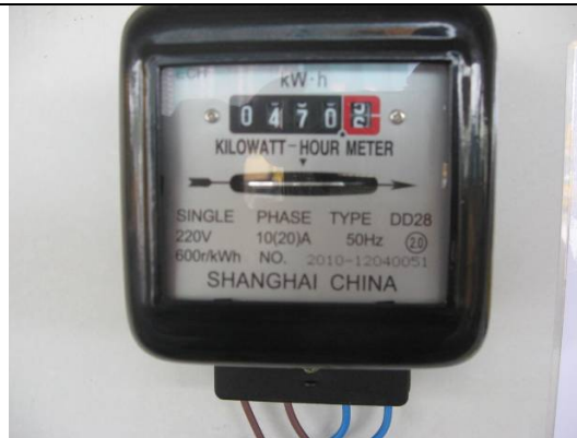
Watt-hour meter of EV-1's charging facility
