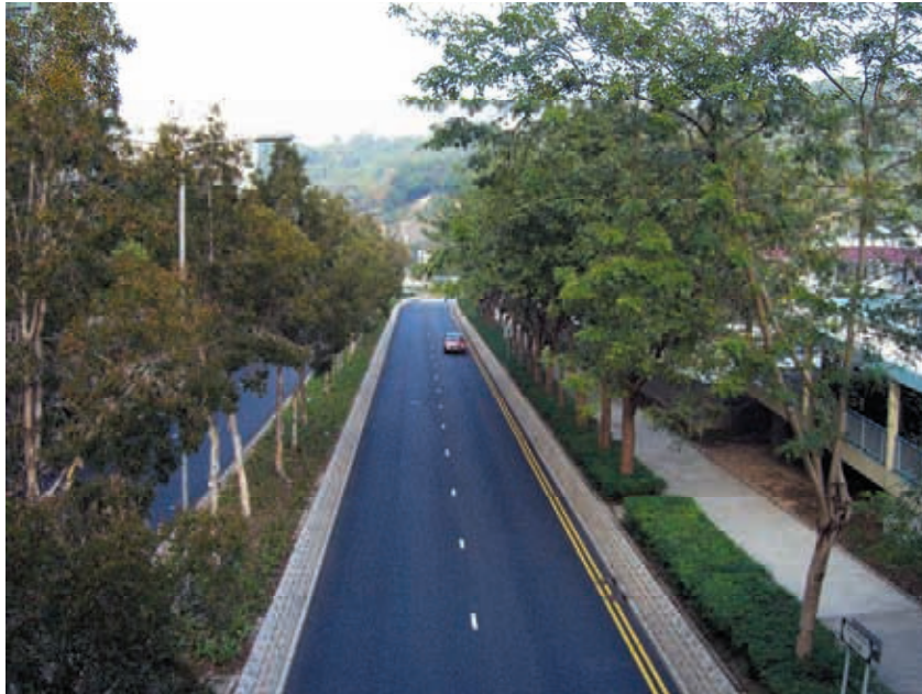
Overlaying low noise road surfacing materials on one of the trial sections
