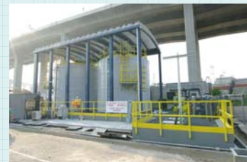
Chemical storage tanks
