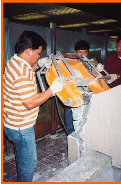
▲ Use of hydraulic crusher can conduct demolition work in a very quiet way
