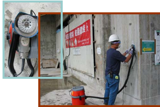
▲ The grinding machine is fixed with the extraction inlet of vacuum cleaner for effective dust control during grinding work
