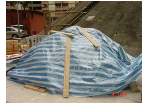
▲ Cover well for dusting materials
