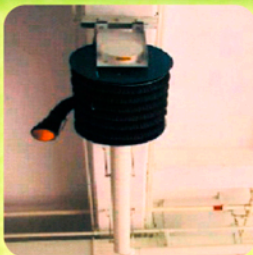
Vehicle exhaust collection facilities
