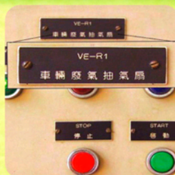
Vehicle exhaust extraction system
