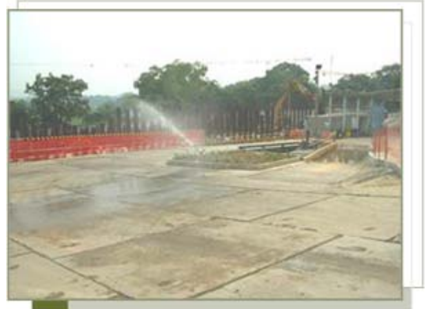
Hard paving construction to reduce nuisance of dust when site vehicles travelling
