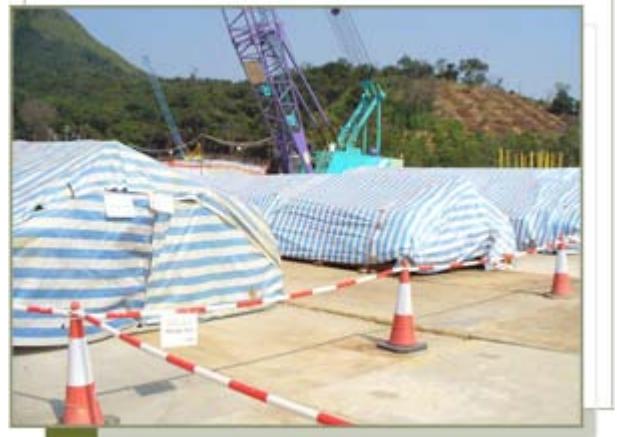
Materials are fully and smoothly covered with tarpaulin sheets. Regular checks are made to identify any undulating surfaces.
