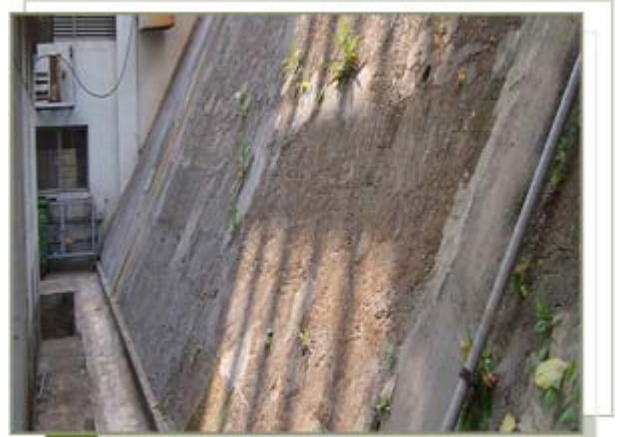
Conduct routine slope maintenance work to prevent vegetation and clear blockage of surface channels
