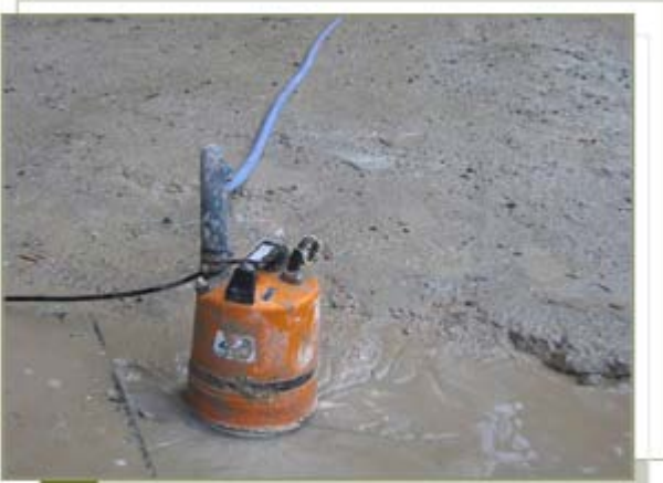
Use of light duty sump pumps to clear stagnant water on the floor
