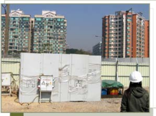
Noise barrier to minimise potential noise impact on a nearby residential area
