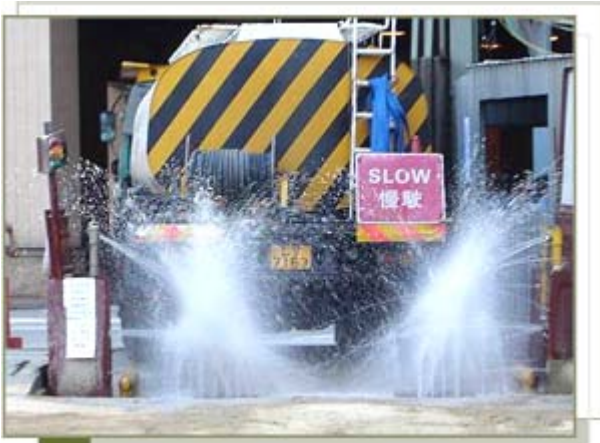
Vehicles leaving the site are first washed to prevent them carrying dirt outside the site
