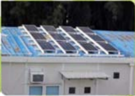
Solar Panel on the Roof 4
