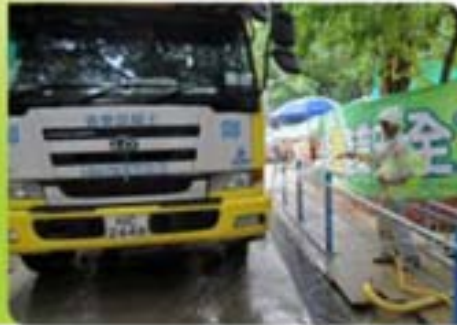
Treated Water Recycled for Wheel Wash 2
