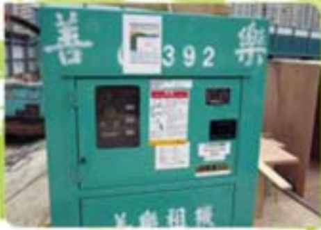
Quieter Quality Powered Mechanical Equipment (QPME) Generators 4
