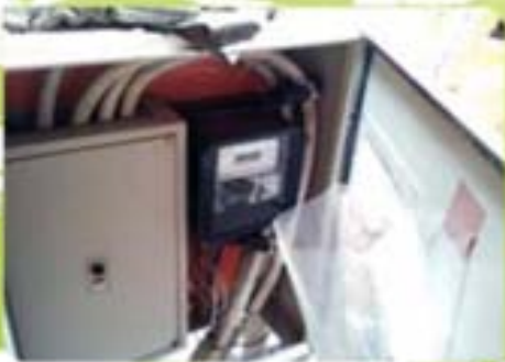
Electric Meter to Monitor Electricity Consumption on Site 6
