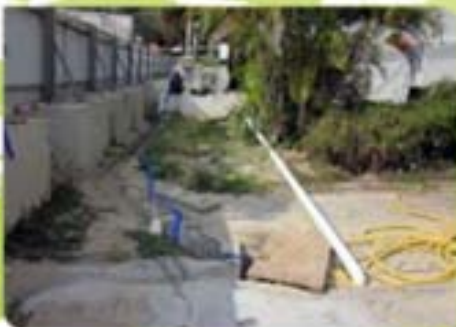
U Channel to Collect Rain Water 4
