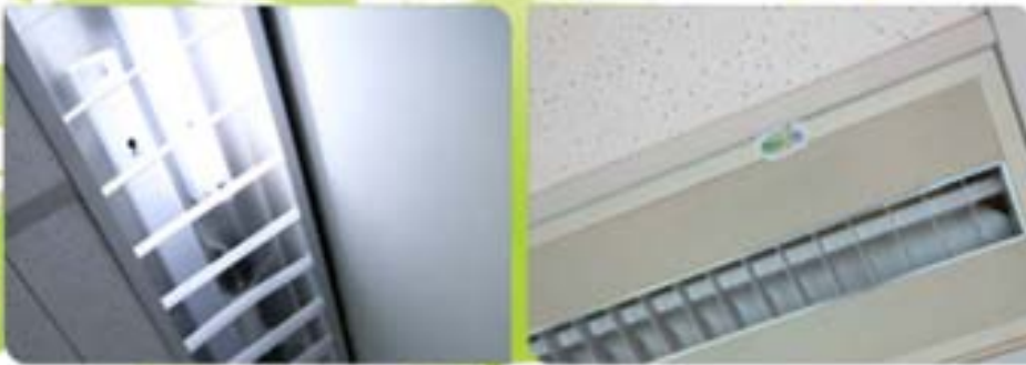
De-lamping of Lighting System to Reduce the Use of Fluorescent Tubes Switch off of T5 tubes
