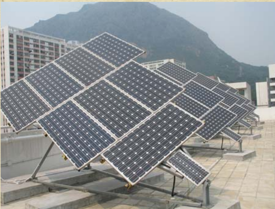
PV Panels with Sun Tracking System
