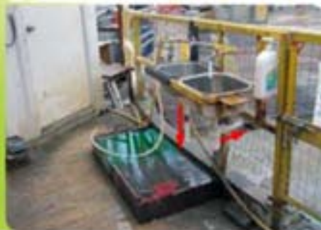
Collect Wastewater for Shoe Washing 3
