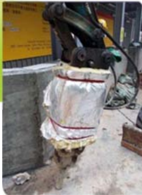
Noise Insulation Jacket on Breaker 3
