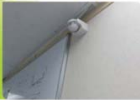
Motion Sensor to Switch off Light when the Room Is Not In Use 3
