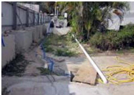
Rainwater collected for watering plant and flushing toilet
