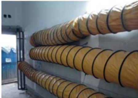
Seal off air duct system to prevent dust and pollutants accumulation
