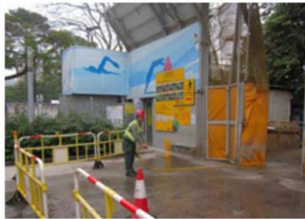
Adopt spray sprinkler system at site entrance
