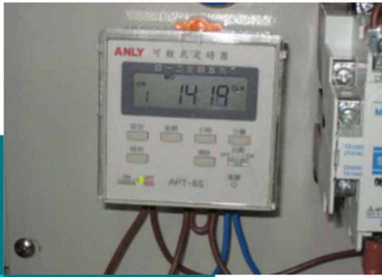
Installation of timer switch for controlling the power supply of non-essential power sockets
