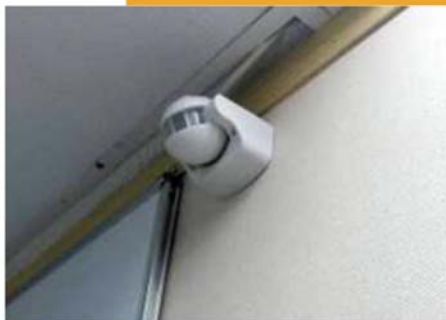
Motion sensor to switch off lighting in meeting room
