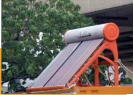
Water heating with solar energy
