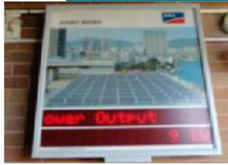
Photovoltaic power production monitoring panel
