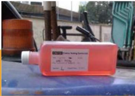
Use Ultra Low Sulphur Diesel (ULSD) with regular testing for fuel on site to reduce air pollution
