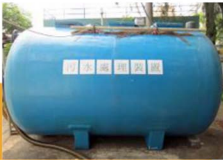
Sewage treatment system
