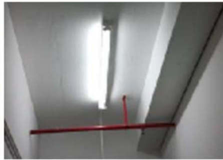
LED lamp with motion sensor installed
