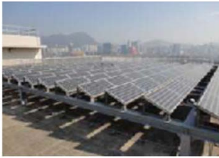
Photovoltaic panels installed on the roof top
