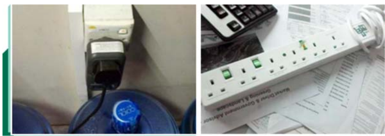
Applying timers for water dispensers
