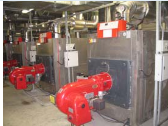
POE site walk to check the operation of condensing hot water gas boilers at New Infectious Disease Block, Princess Margaret Hospital
