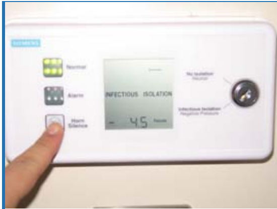
POE Team checking the differential pressure condition of isolation rooms and anterooms during site walk
