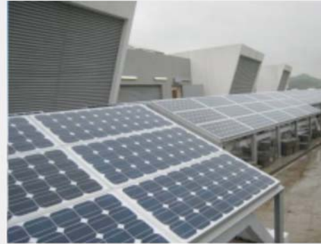
Photovoltaic panels for electricity generation
