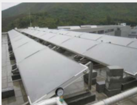
Solar panels for hot water preheating at Central Block
