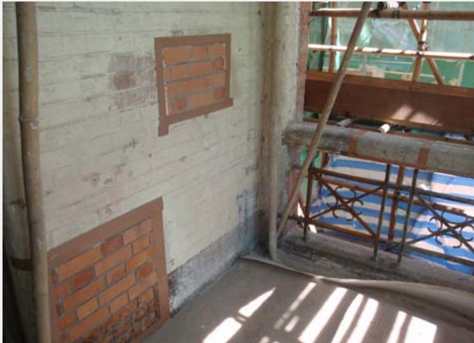
Small area of the brickwork was restored to evaluate the condition of the brickwork. (Yau Ma Tei Theatre Red Brick Building)
