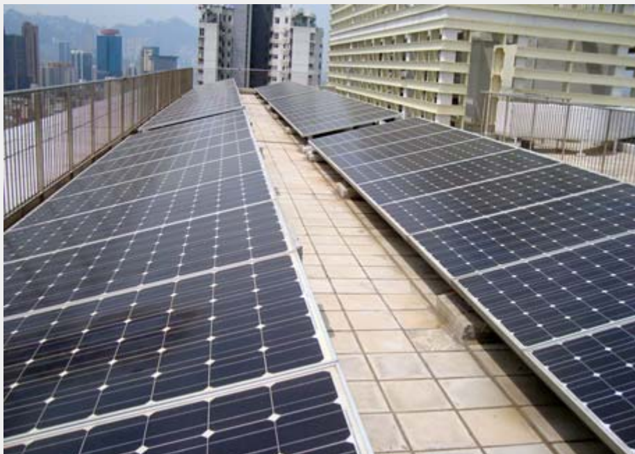
Photovoltaic Panels at Roof for Electricity Generation
