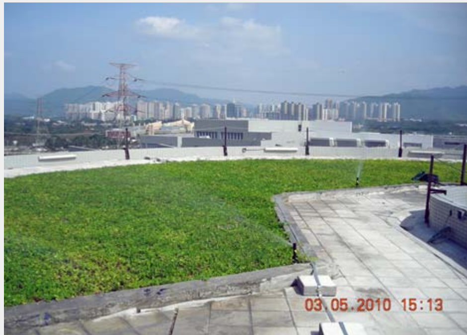
Watering grasses through grey-water recycling system in Lo Wu Correctional Institution
