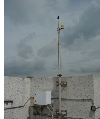
Figure 2-3: Outdoor Noise Monitoring Terminals
