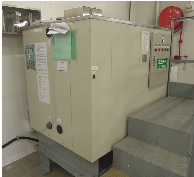
Figure 5-14: The food waste decomposition system in CAD Headquarters
