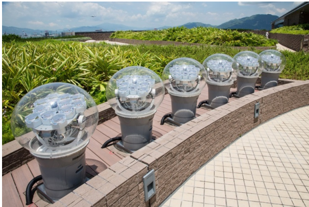
Figure 5-2: Solar Light Collectors with Fiber Optics (tracking feature installed)
