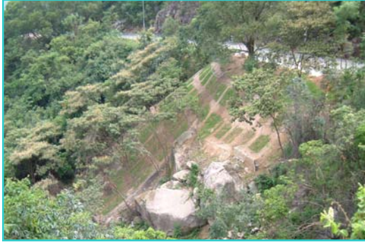
As-built photo taken in August 2003, concrete grill structure can be seen from distance.
