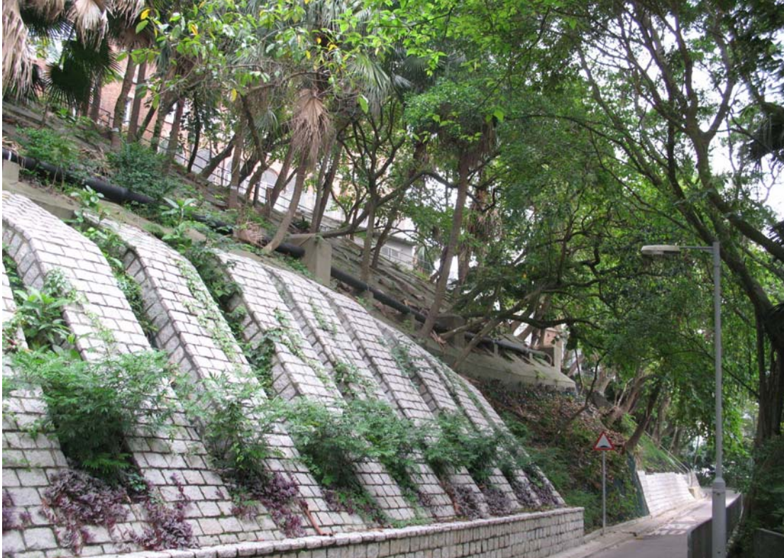
Landscaping work on an LPM slope along Bowen Road shows tree preservation, hard landscaping and at the same time maximizing planting opportunity.
